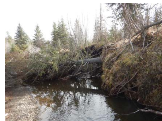
Plate 12: Unstable and slumping bank at transect 14. 22 October 2014
