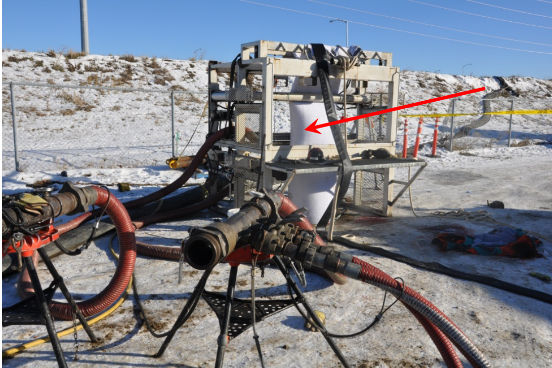
Figure 1. Dual Gland Air Inversion (DGAI) Unit located in alley beside 129 Cranberry Square, Calgary, Alberta the day of the incident. The photo shows the liner (indicated by arrow) in place in the DGAI Unit.
