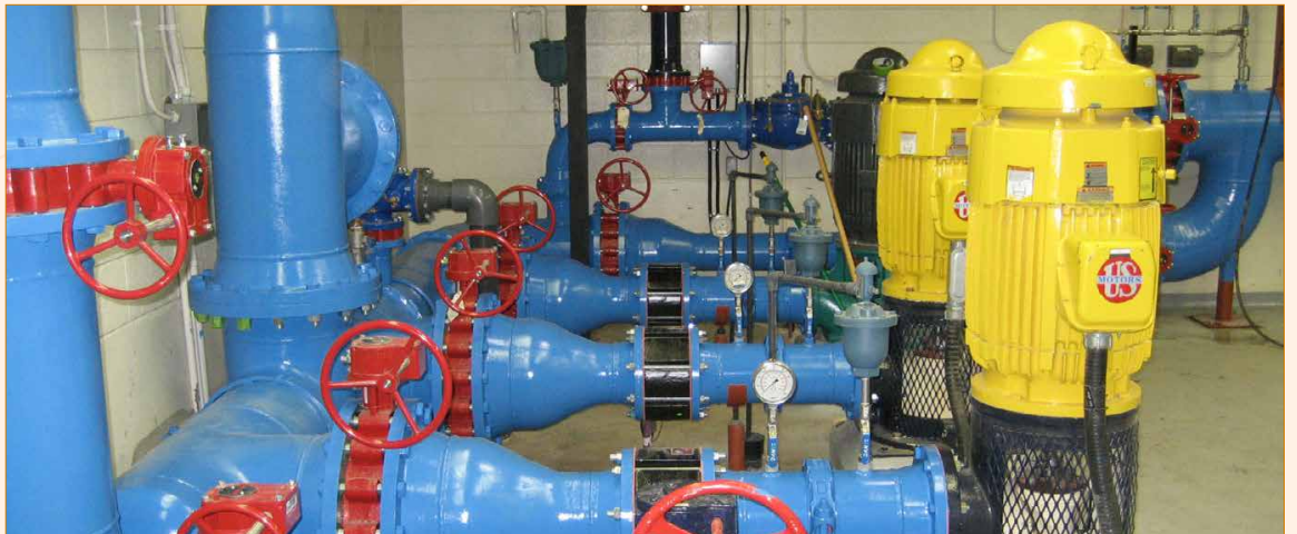
Capital Region Northeast Water Services Commission, Mechanical Equipment at OLPS
