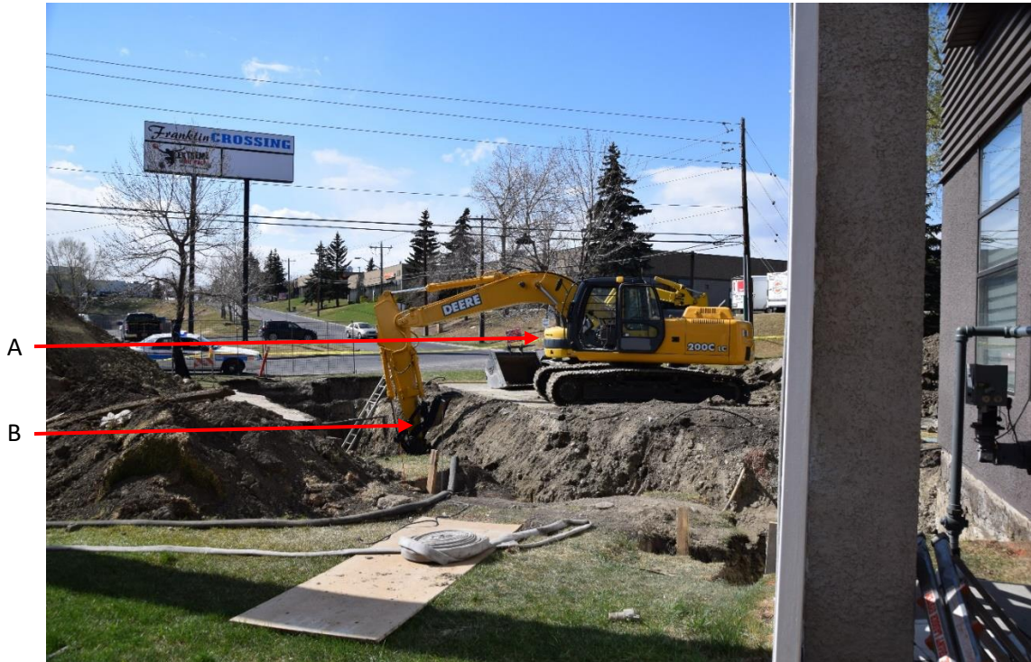
Figure 1. The excavator used by RM at the incident location on or about April 15, 2016. The excavator was used in the excavation of the water line.
