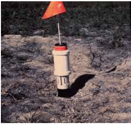
Slow release drop structure Inlet.
