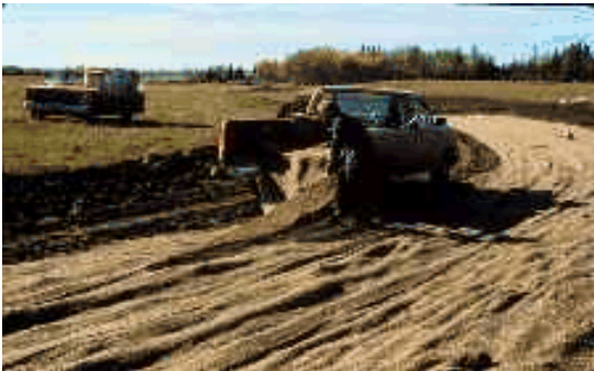
A newly constructed waterway may need protection until the grass cover is established.
