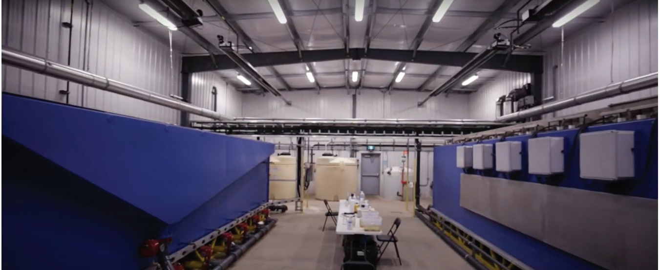
Town of Sundre Wastewater Project
