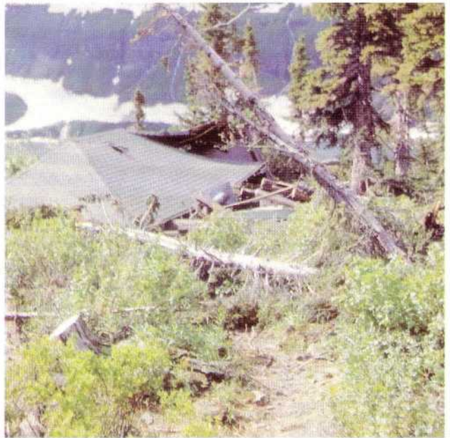
Figure 76. Damage to a picnic shelter located at the bottom of a Chute.
