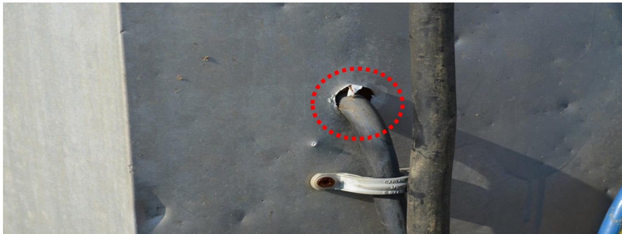
The red circle indicates the black cord run through the wall of the trailer.
