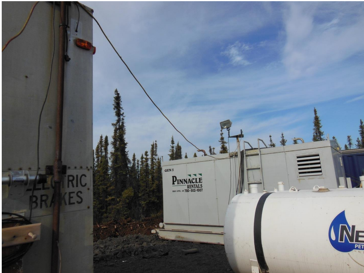
Pinnacle Rentals Stamford AC Generator Set the main electrical source (generator unit 5).
