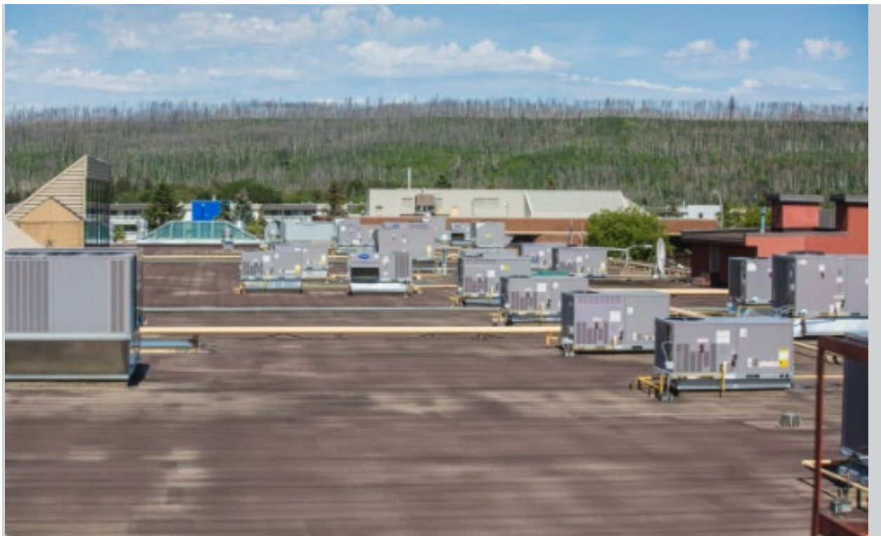
A large HVAC replacement on the roof kick-started the mall's electricity savings.
