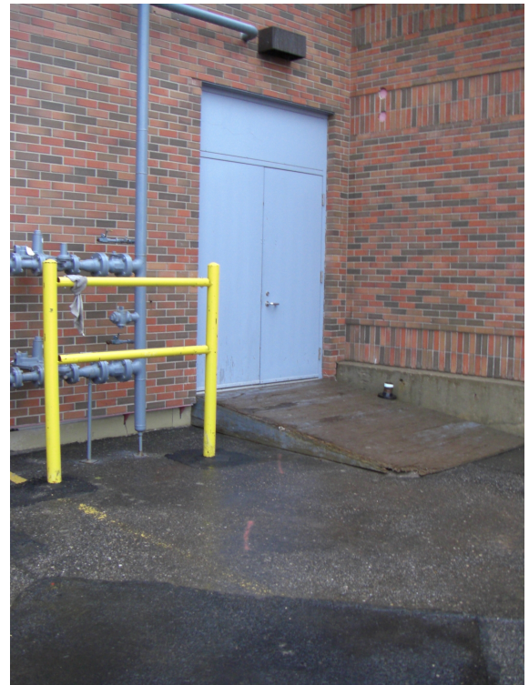
(1985) Basement (Maintenance - Mechanical Room 0160) - wood ramp is worn out.
