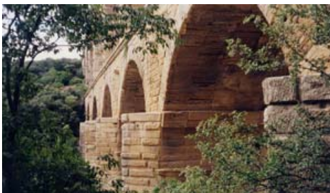
Pont du Gard Bridge near Nîmes, France (18 BC) (For description, see Dupré, 1997)
