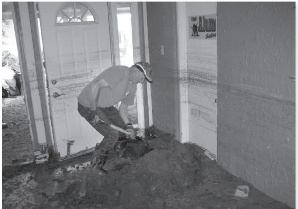
A volunteer removing mud from the interior of a house (notice the water-line on the wall).
