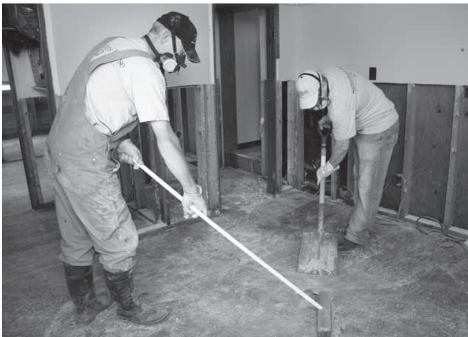
Interior of a house after Samaritan's Purse volunteer clean up teams have completed a mud-out.
