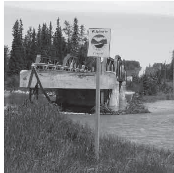
A bridge along the James River that was washed out during the flood event (June 2005).
