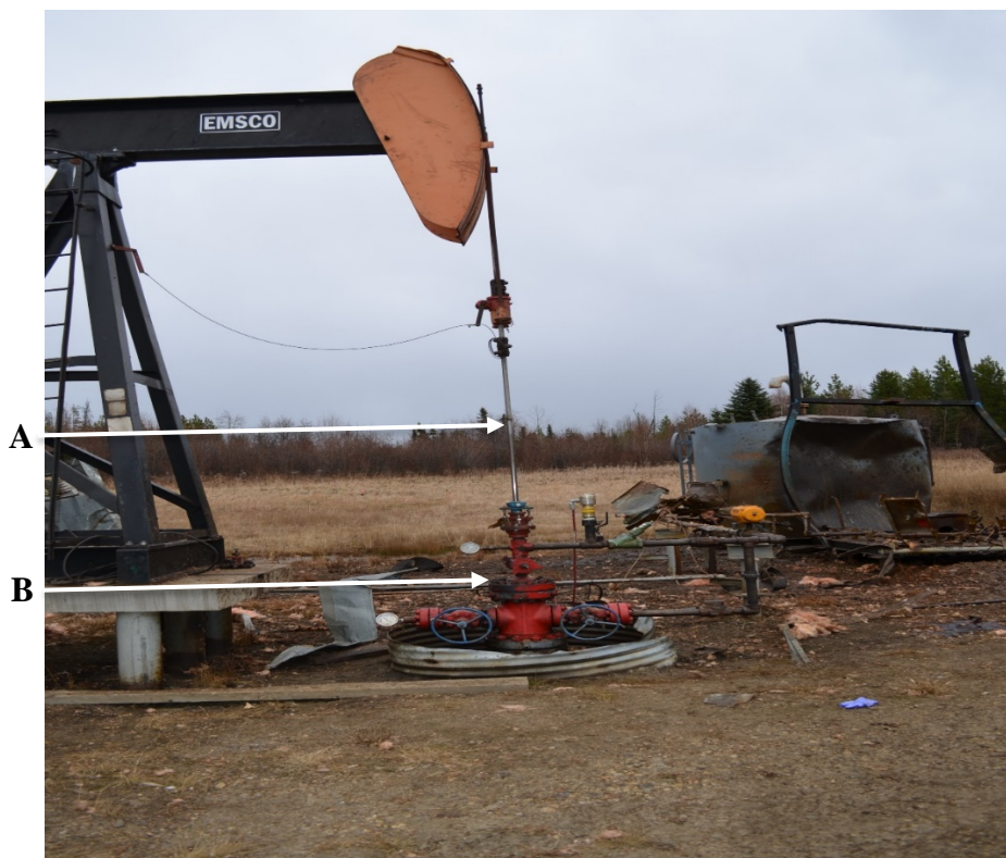
Figure 1. The wellhead and pumpjack sucker rod system still intact post explosion.
