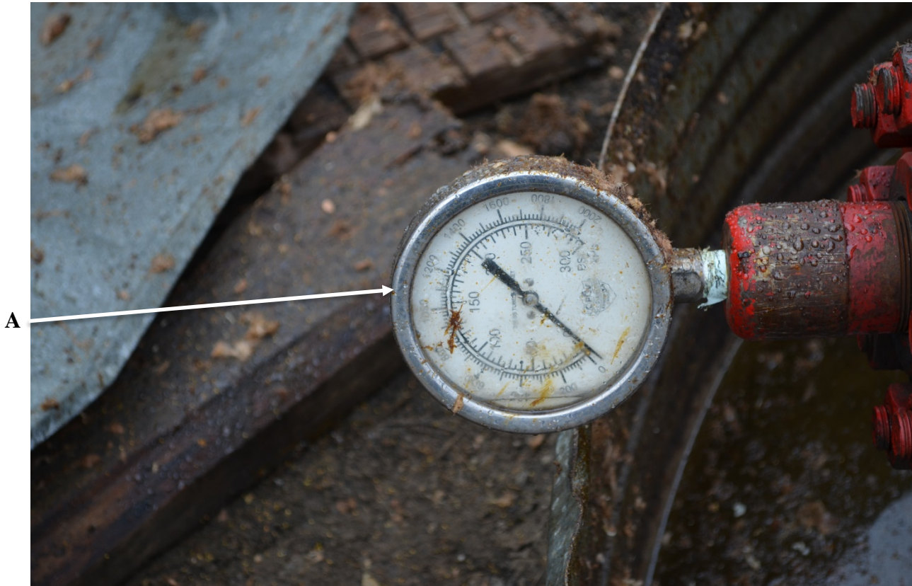
Figure 3. The pressure gauge needle was wrapped around the gauge and was sitting below the “0”. This was caused by a pressure, beyond the pressure gauge’s capacity of 300 pounds per square inch (psi), coming from down hole and through the piping that the pressure gauge was attached to.
