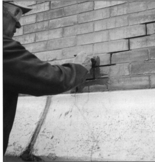
Figures 8 & 9: The final step in joint preparation is to ensure that all loose mortar has been removed. Here the joint is first brushed out and then rinsed with water.
