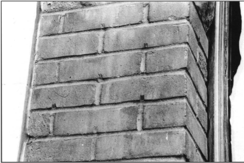
Figure 5: Damage caused to brickwork by a circular saw used to remove mortar from the vertical joints.
