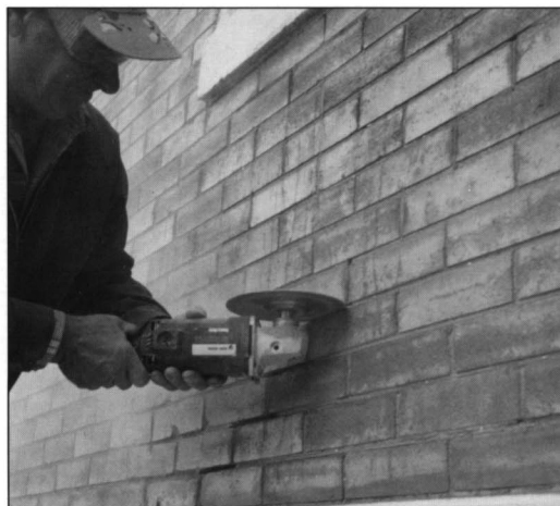
Figures 6 & 7: In the hands of a skilled mason, a circular saw may be an effective tool for mortar removal. In this repointing project at a Provincial Historic Resource, mortar replacement was necessary to repair a series of cracks which had opened as a result of nearby construction. As the mortar itself was relatively hard and sound, use of the power tool was allowed, but restricted to the horizontal joints. Mortar from the vertical joints was removed using a chisel. [Charlie Wildermann of Pockar Masonry (Northern) Ltd., working on Old St. Stephen's College, Edmonton.]
