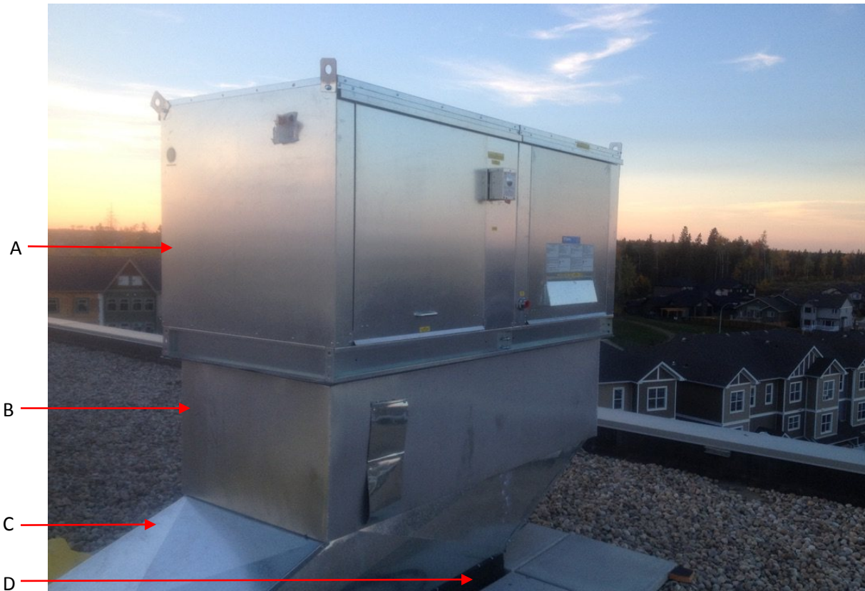
Figure 1. MAU with offset curb pre-accident (photo provided by Marathon Ventilation).
