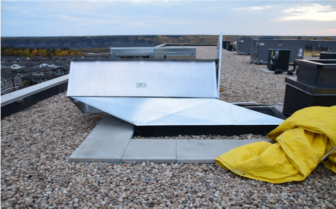
Figure 2. Offset curb with manufactured curb post-accident.
