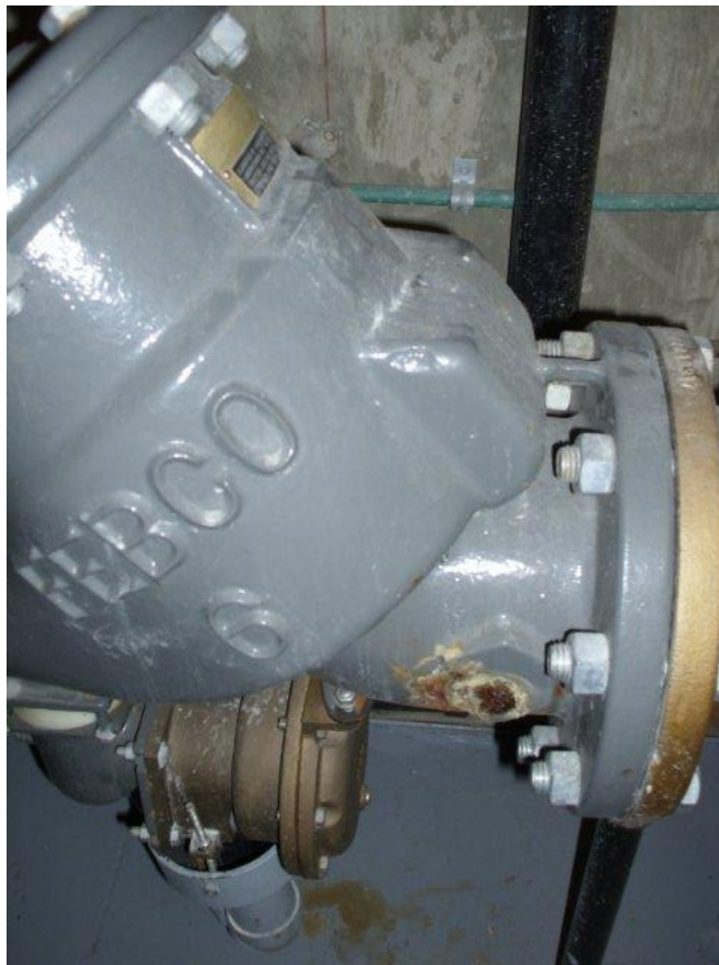
Backflow preventer with location requiring regular repairs (rusty spot near flange).
