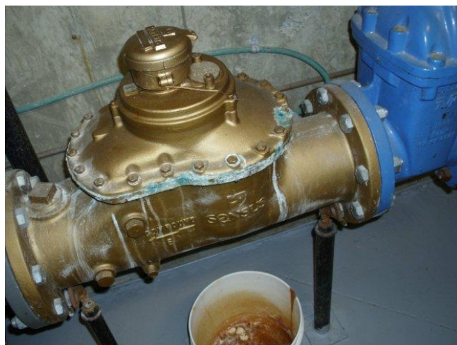
Leaking seal at main water meter.
