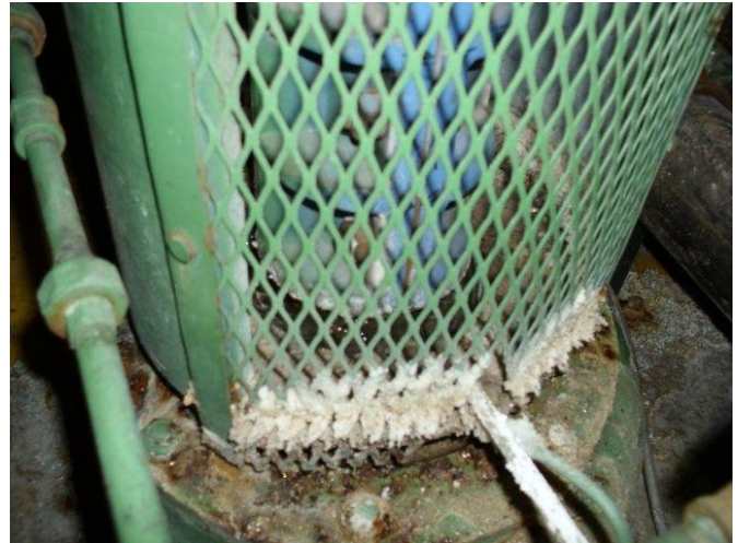
P22 leaky seal
