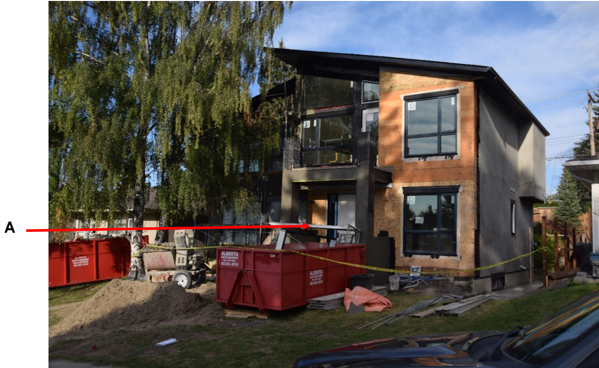
Figure 1. The front of 104 Cheyenne Crescent NW, Calgary, Alberta. A. The incident scaffold, work area and incident location
