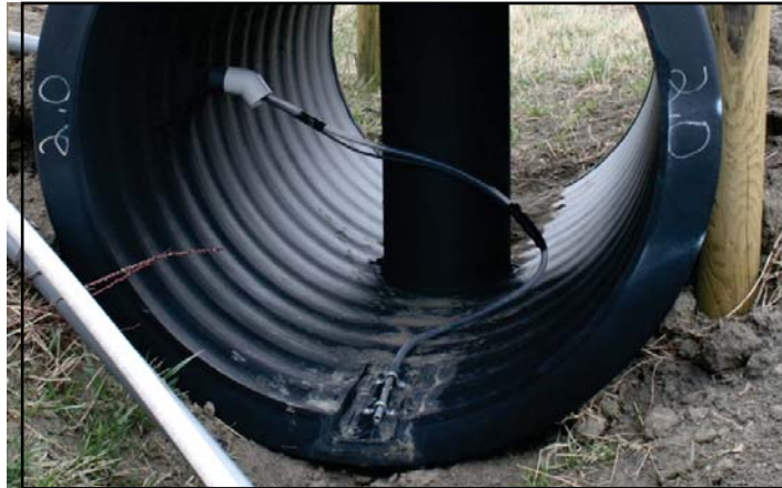
Figure 2.23. Isco intake line in the trough at bottom of a circular flume.
