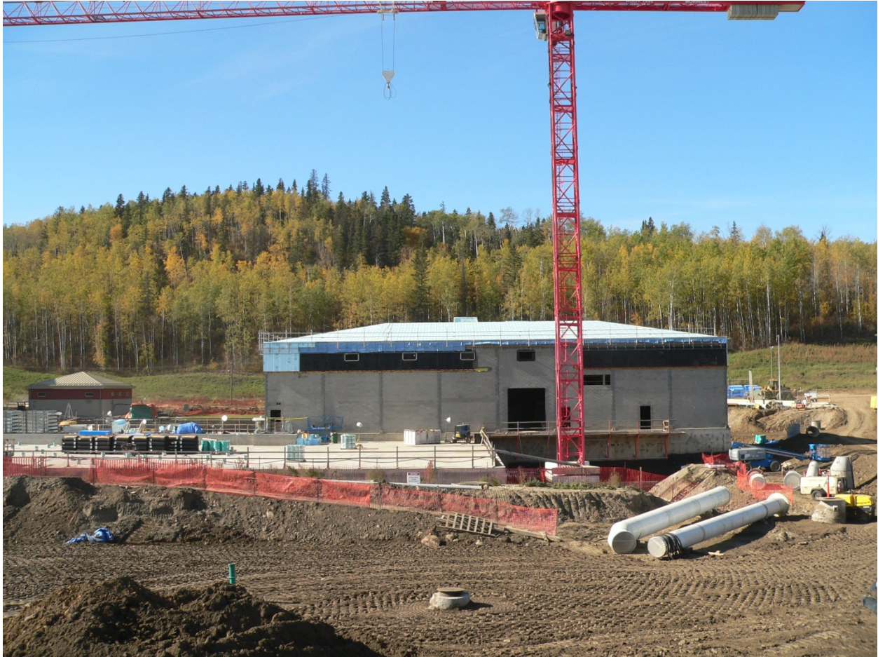
Figure 1 – High Lift Pump Station (HLPS)
