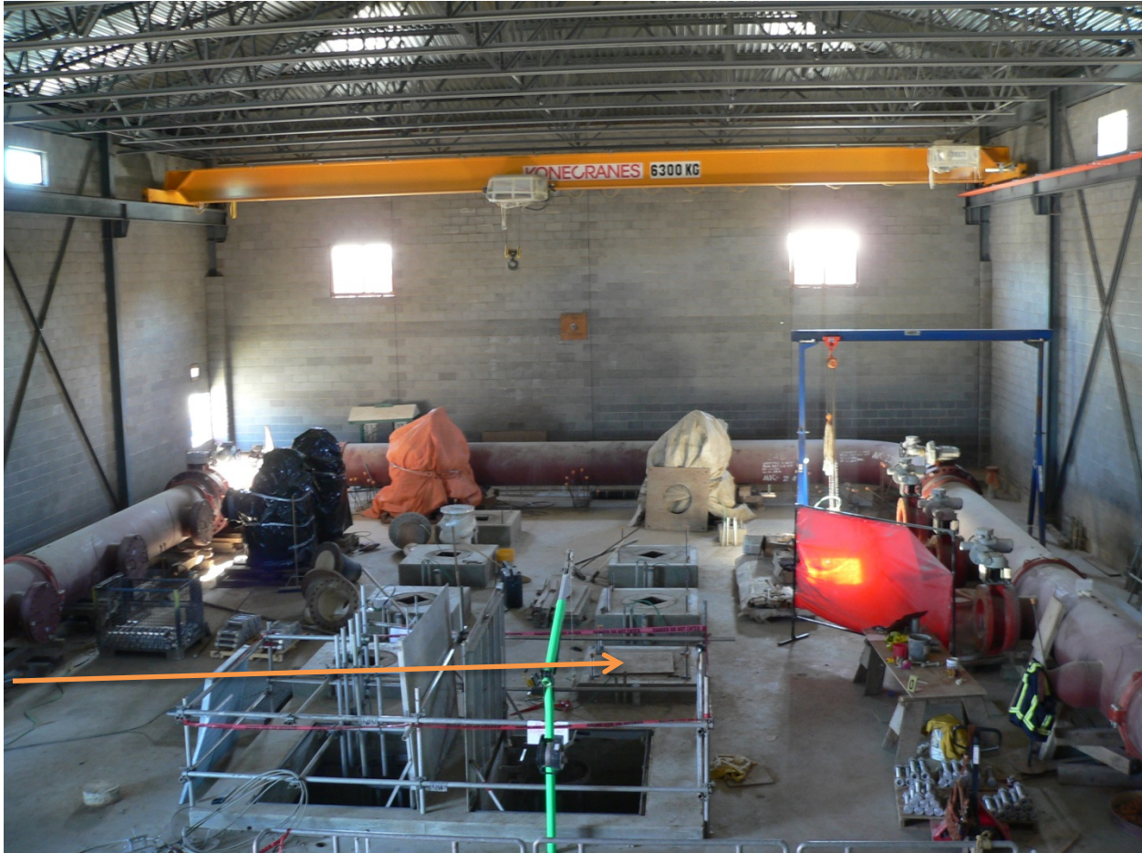
Figure 4 – Inside of the HLPS where the pump bases were located.
