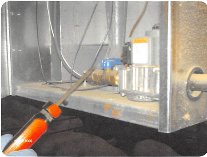
Figure 2. Adjusting the gas valve on some forced air heaters provides more efficient fuel use and helps maintain a steady barn temperature
