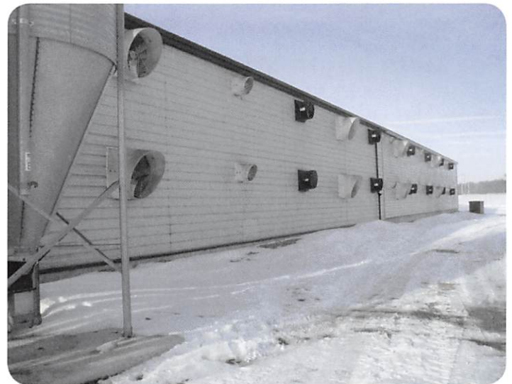
Figure 3. Careful placement and sizing of fan stages is essential for proper ventilation systems performance
