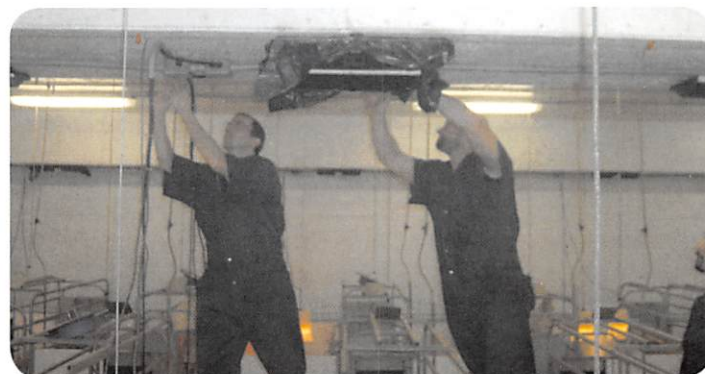
Figure 1. Calibration and adjustment of air inlets
