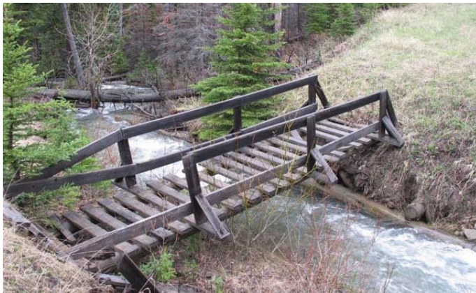
An old bridge that has fallen to disrepair. This is a hazard and a liability.
