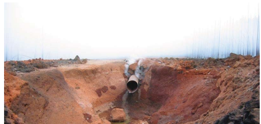
This is an image of an exploded pipeline.
