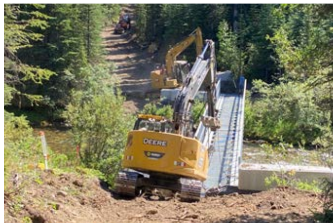
New bridge construction at MacKenzie creek helps keep "wheels out of water" on the new trail.
