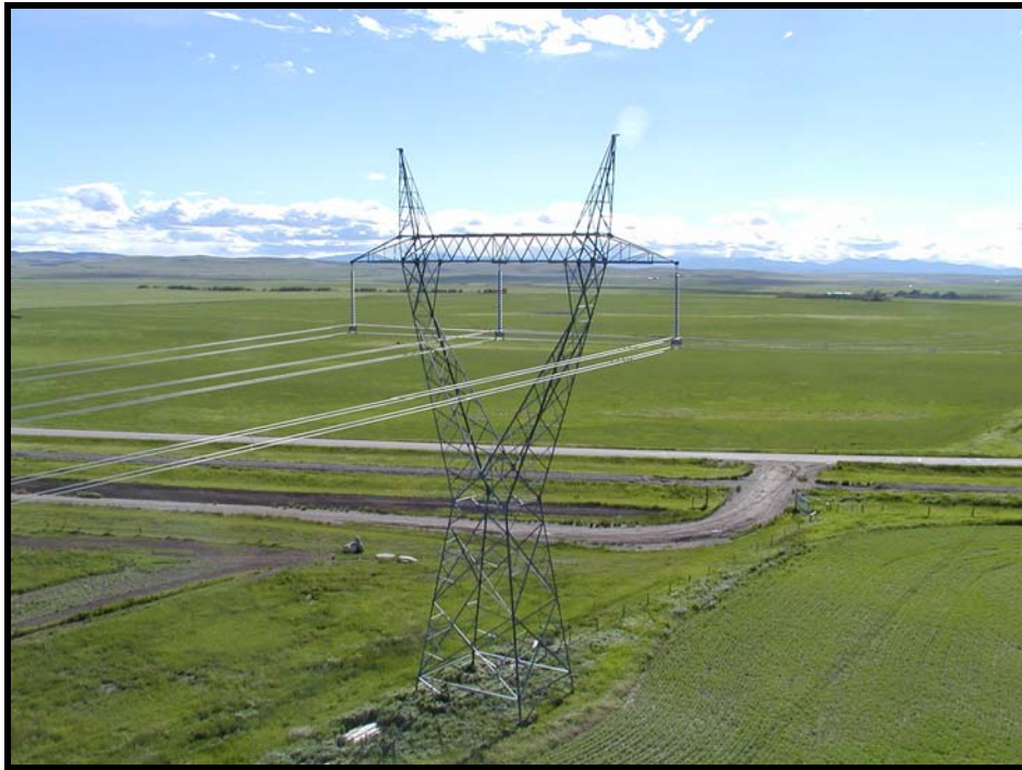
500 kV Tower – 7.67 m x 6.11 m (1202 L).
