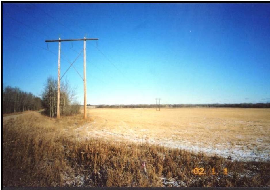
138 kV H-frame – 6.1 m apart (80 L).
