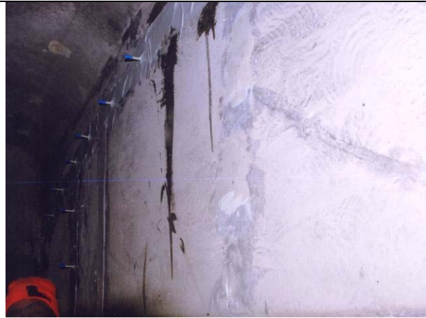
Following curing of the epoxy resin, ports and crack sealant shall be completely removed.
