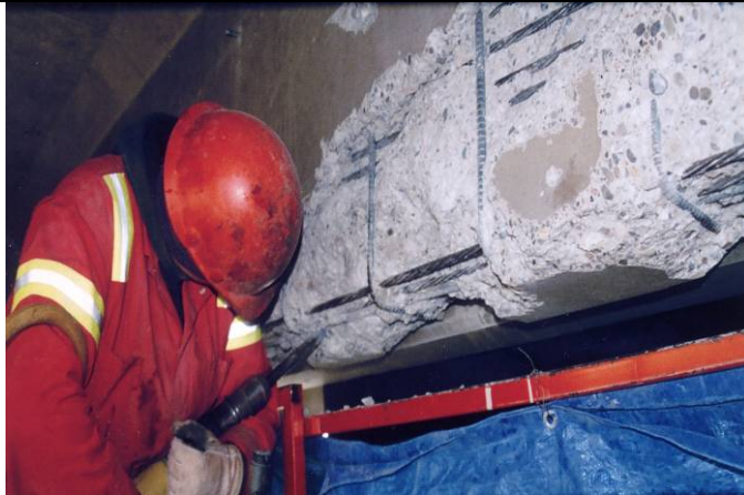
Loose, delaminated concrete shall be removed using small tools – care exercised to ensure that prestressing strands are not damaged.
