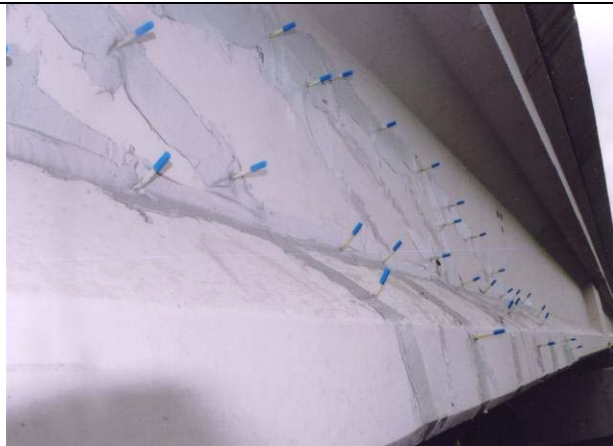
Cracks shall be temporarily sealed and injection ports installed – spacing of the ports shall be maximum 150mm.
