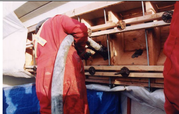
Pumping concrete into plywood formed leg section. Spacing of pour access holes shall not exceed 600mm.
