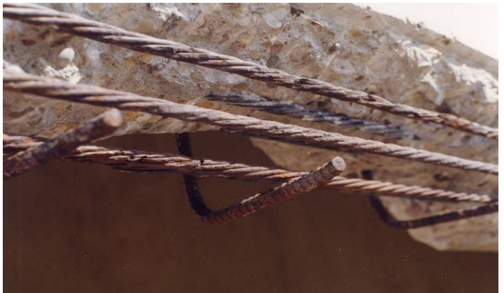
The effects of corrosion damage can result in loss of prestressing forces.
