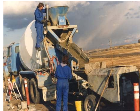
Transit mix and concrete pump. Concrete must be placed, pumped within 70 minutes of being batched.
