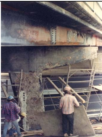
Rebound hammer and core testing is performed to determine the extent of fire damage.
