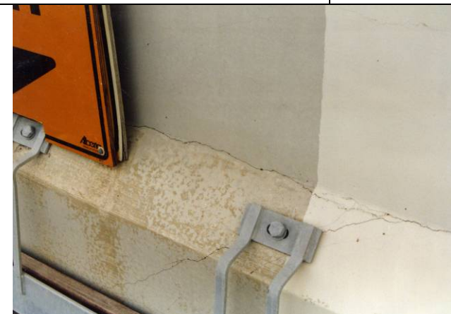
Cracks in concrete sections \geq 0.3 mm shall be full depth pressure injected with approved epoxy resins.
