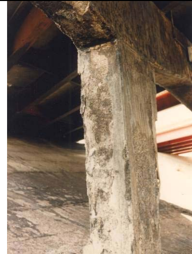
Delamination sounding may be required on concrete elements. Hardness testing will aid to determine the extent of severe damage.
