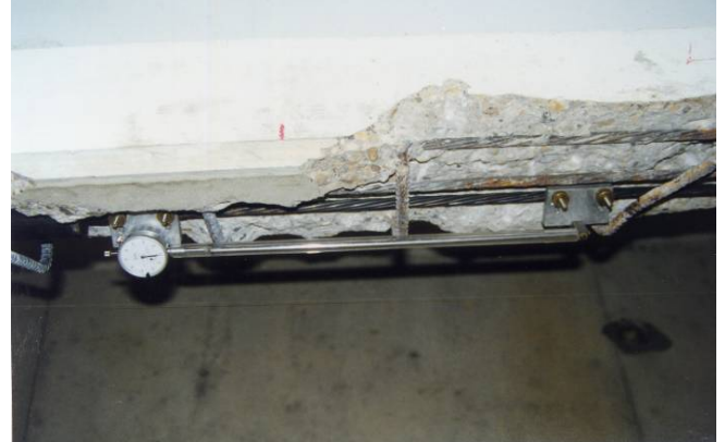
Strand repair tension loads are applied to initial design values using dial gauges and devices to monitor elongations at accuracy of 1/1000 of an inch or 0.100”.
