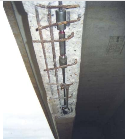
Strand corrosion damage restored. Determine the extent of damage, splice and tension strands.
