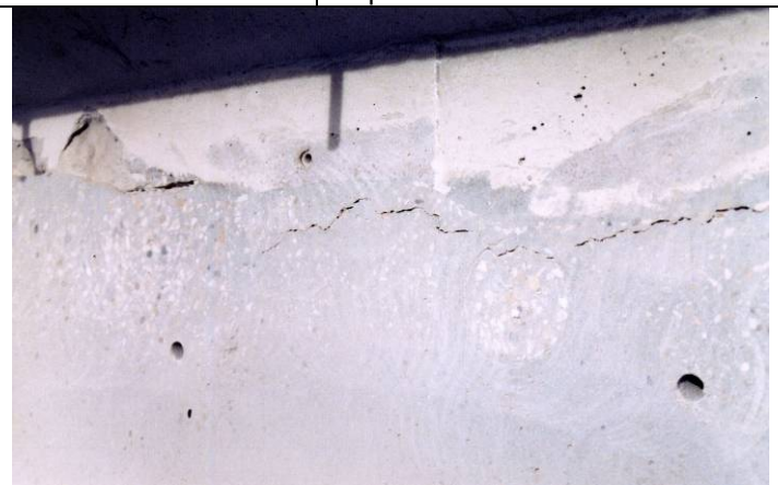
Pour / cast perimeter lines shall be full depth pressure injected with epoxy resins.
