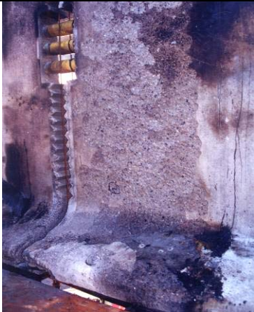
An assessment is required when concrete components have been damaged by fire. The color of concrete may indicate maximum exposed temperatures.
