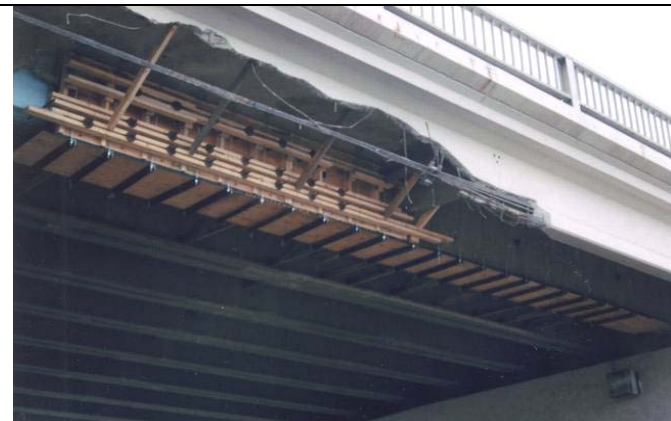
Damaged portions of girders shall be recast to restore the original lines. Forming shall be new plywood materials such as “Coated Formply” Evans 107, or approved equivalent – or steel forms.
