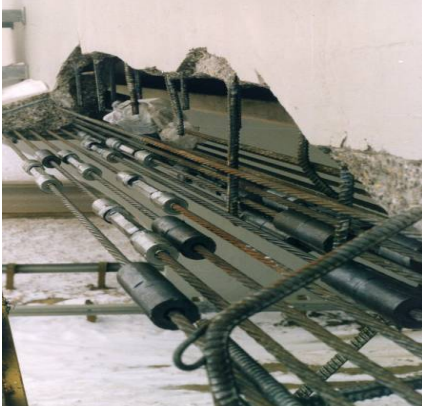
Damaged strands shall be spliced and re-stressed to initial design tension of 128.5 kN. Splices shall be staggered to avoid congestion.
