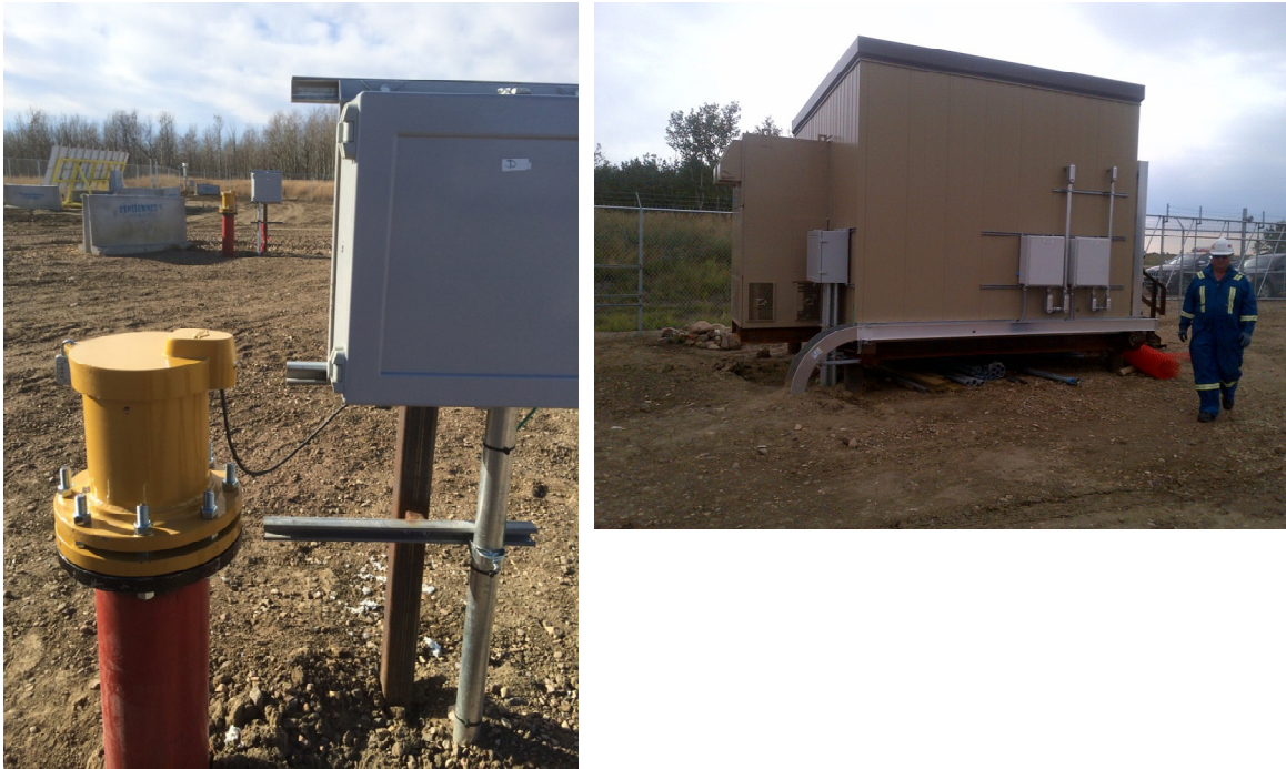
Figure 6-9: MMV infrastructure – Groundwater well surface interface equipment (left) and MMV building (right)
