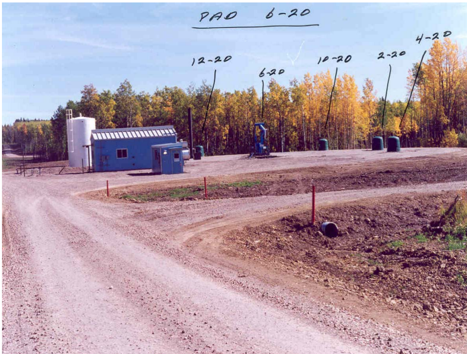
Vertical oil well with slant water wells with production facilities
