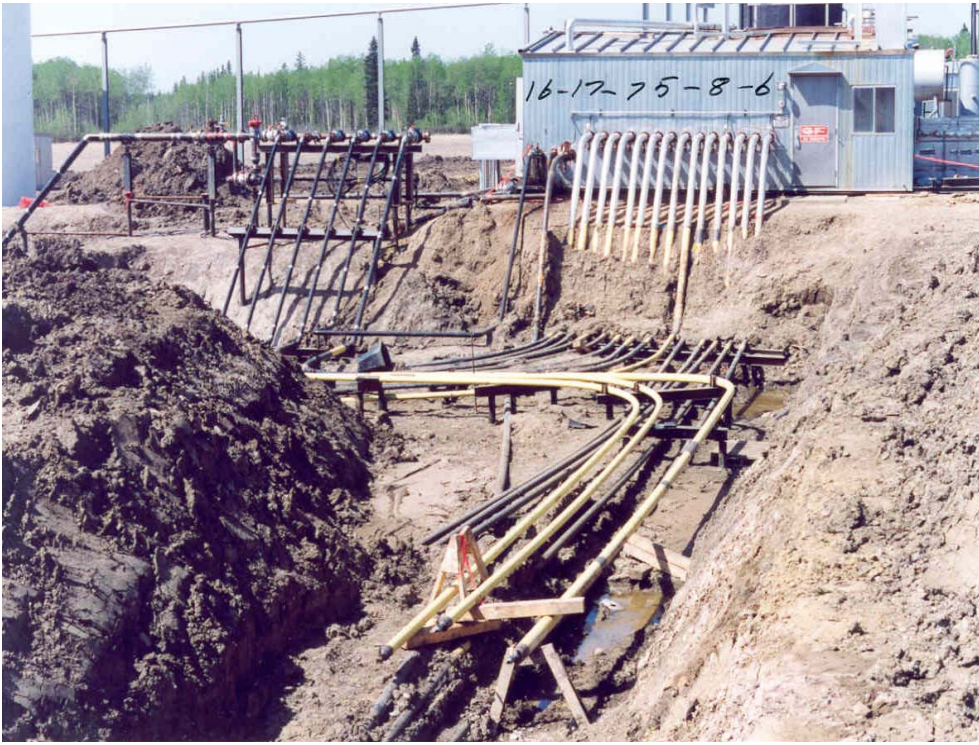
Underground facilities may impact well positioning
