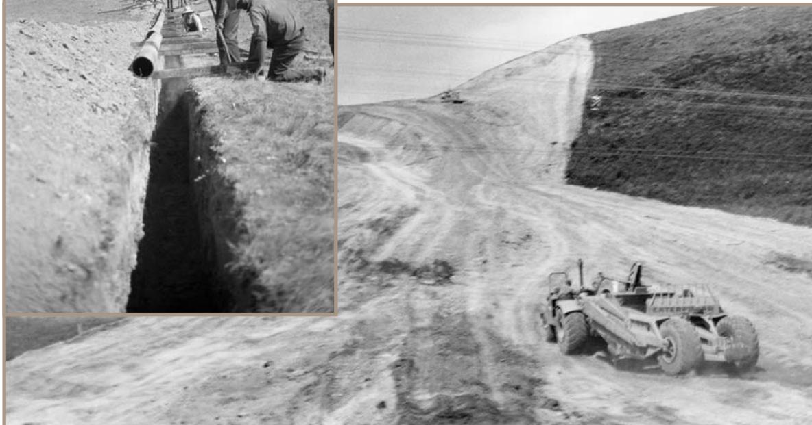
Earthmover working on CP Railway Spur Line 11 Miles South of Pincher Creek, Alberta, 1961
