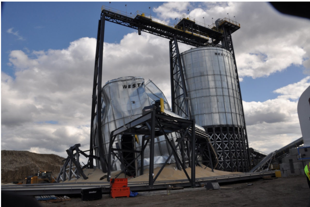
Figure 5. Collapse of bin 2.
