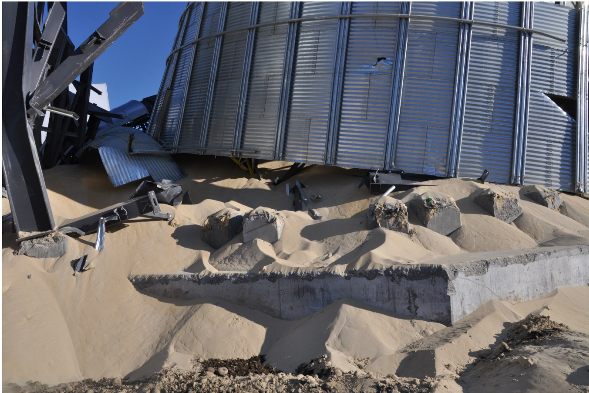
Figure 6. Collapse of bin 2 where the sand ejected through to the bottom hopper panels.
