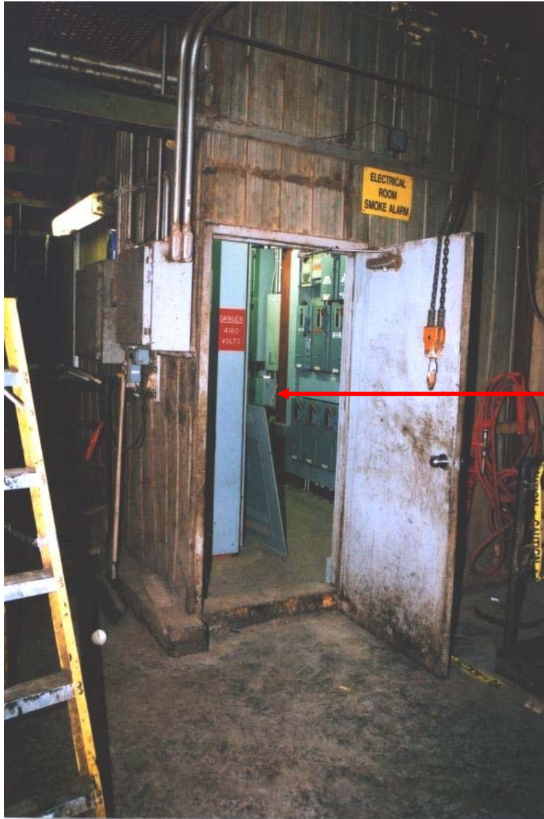
Photograph 2: Arrow shows the entrance door to the electrical room.
