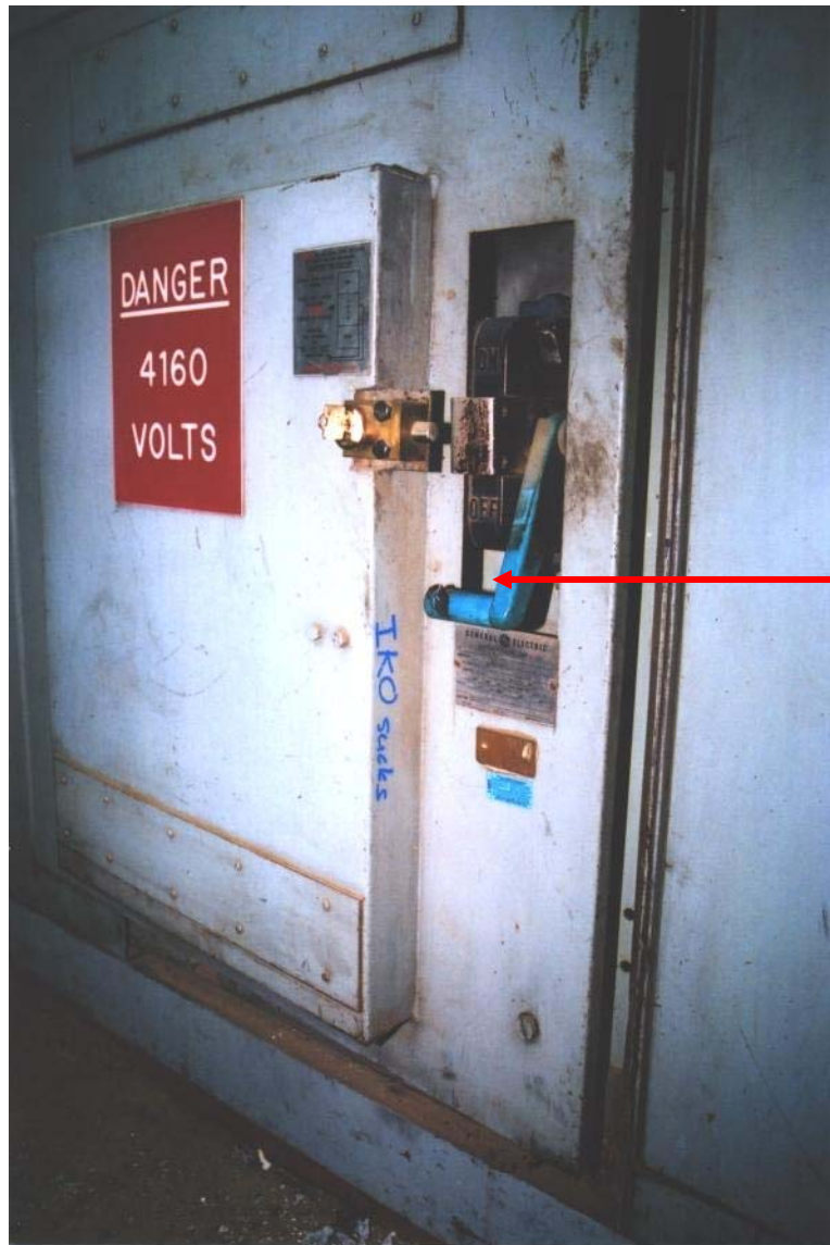
Photograph 4: Shows the high voltage of 4160 volts compartment of the GE Limitamp enclosure.
