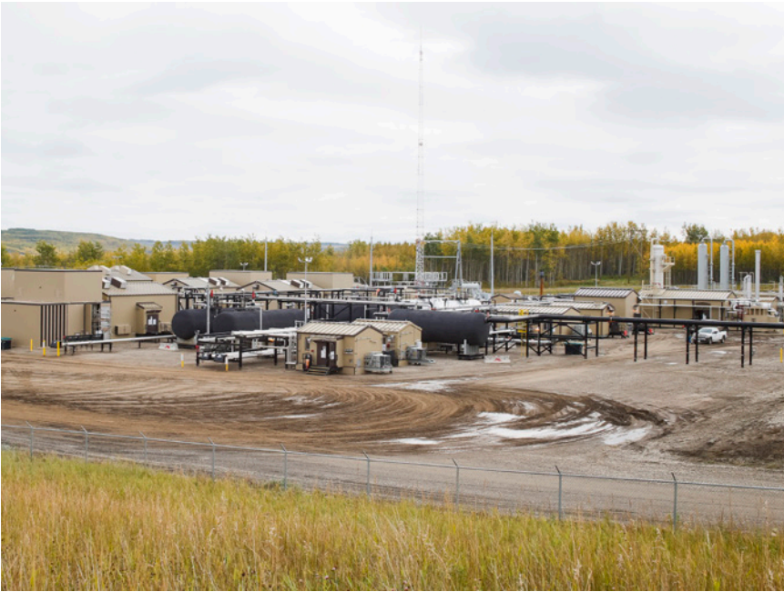
A MONTNEY PUMP STATION OPERATED BY ENCANA.
