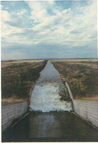
Above: This small spillway located east of Taber, Alberta is part of the irrigation system vital to the agricultural industry in Alberta. Funds are being provided in order to increase Alberta's capacity to produce food and to further diversify its agricultural industry.
