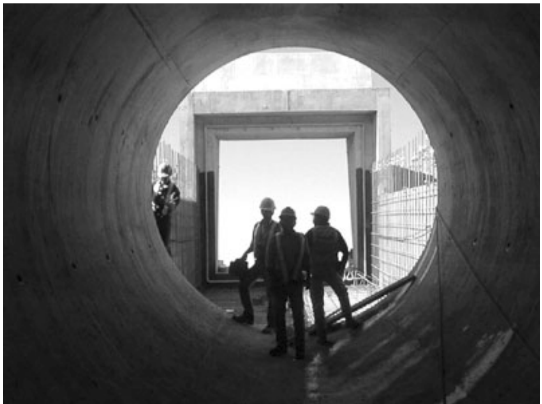
Replacement of the East Arrowwood Syphon on the Carseland-Bow River Headworks System, 25 km southeast of Carseland and 40 km north of Vulcan. The syphon conveys water from the main canal across the East Arrowwood Creek valley.
