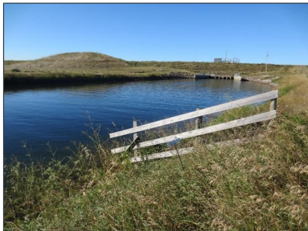
Outlet of Little Bow Reservoir into Bow River Irrigation District Main Canal
