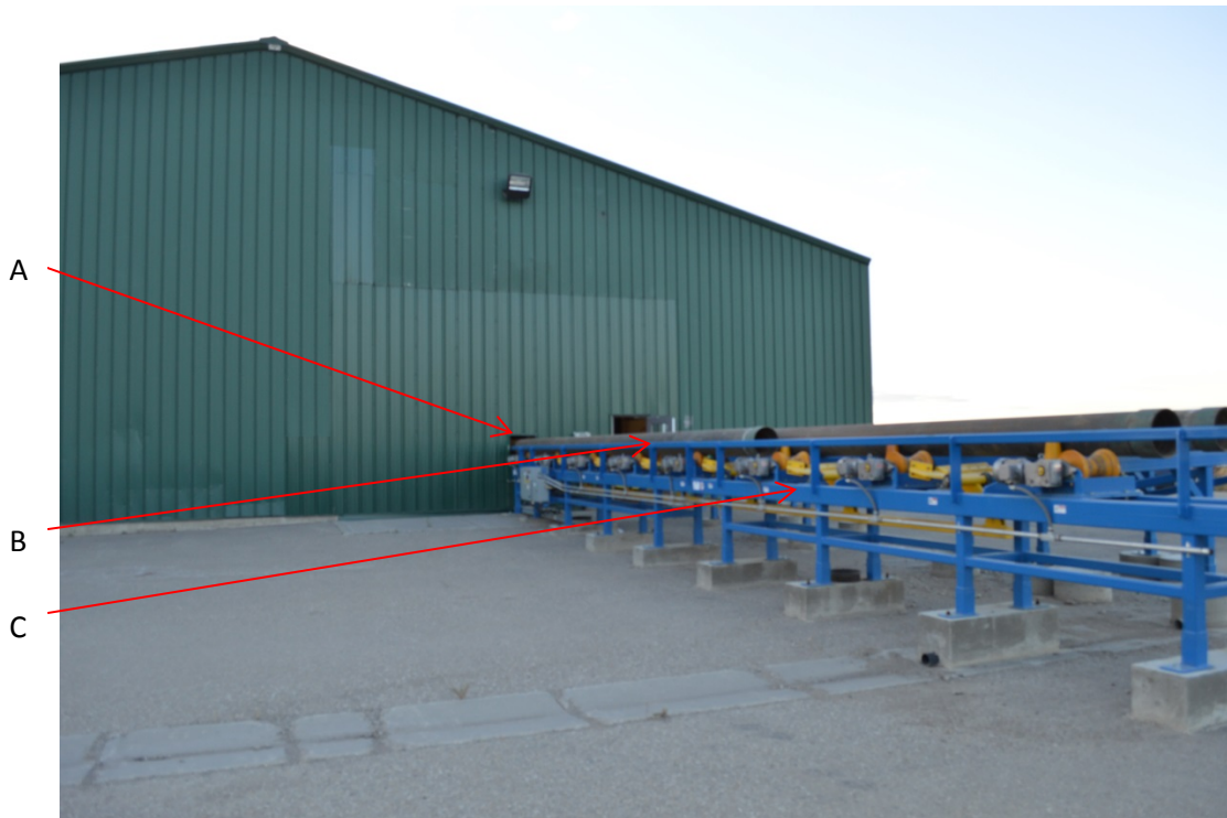
Figure 4 shows C1 conveyor that had a pipe that had been kicked onto the conveyor and brought into the building through the hole in the wall by the controls that were in “auto.” A-Shows the opening used to move pipes into the building using conveyor C1. B-Shows the pipe that was involved in the incident. C-Shows C1 conveyor that had the pipe that was kicked onto conveyor C1 from the pipe stand while in “auto” mode.
