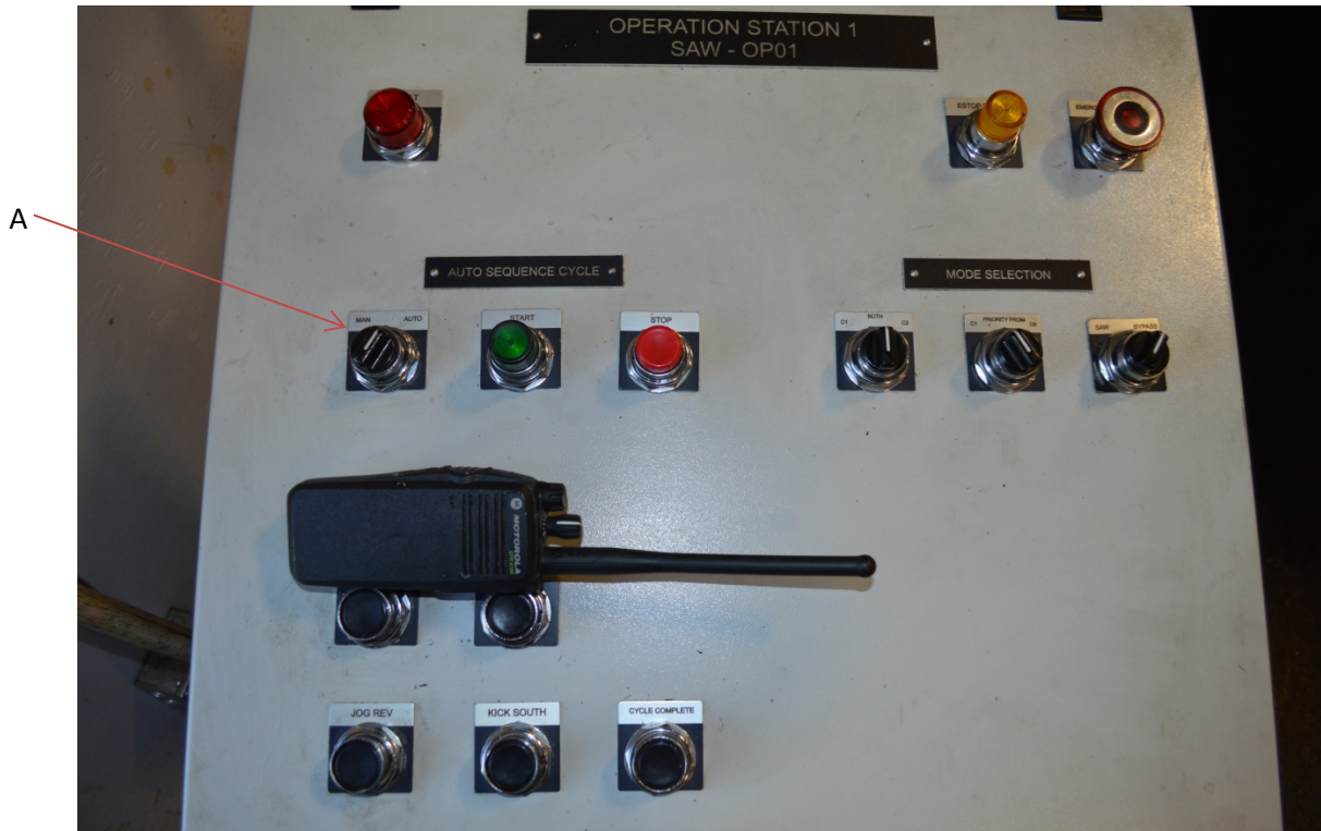
Figure 2 shows the controls for the pipe conveyor system. A-shows the conveyor set to “auto” mode.
