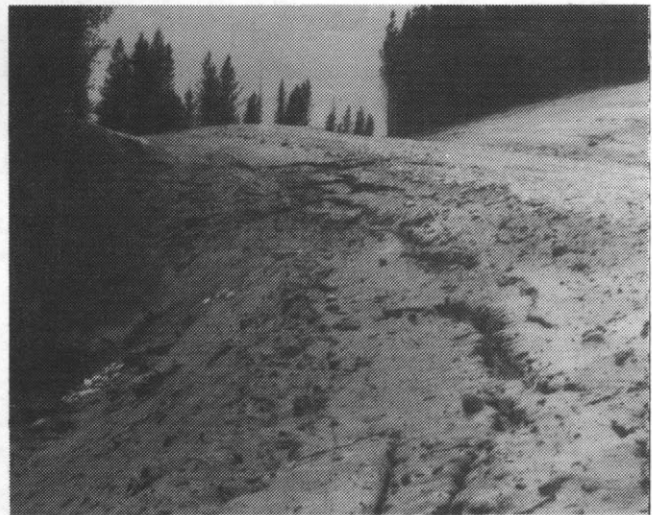
PLATE 17. Very sandy soils tend to be unstable in deep road fills.
