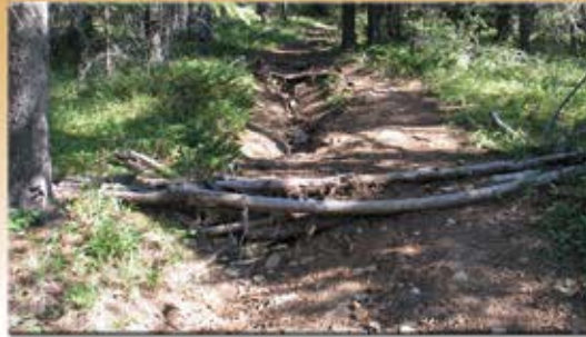
Soil erosion on the left side of the trail, due to water channelling
