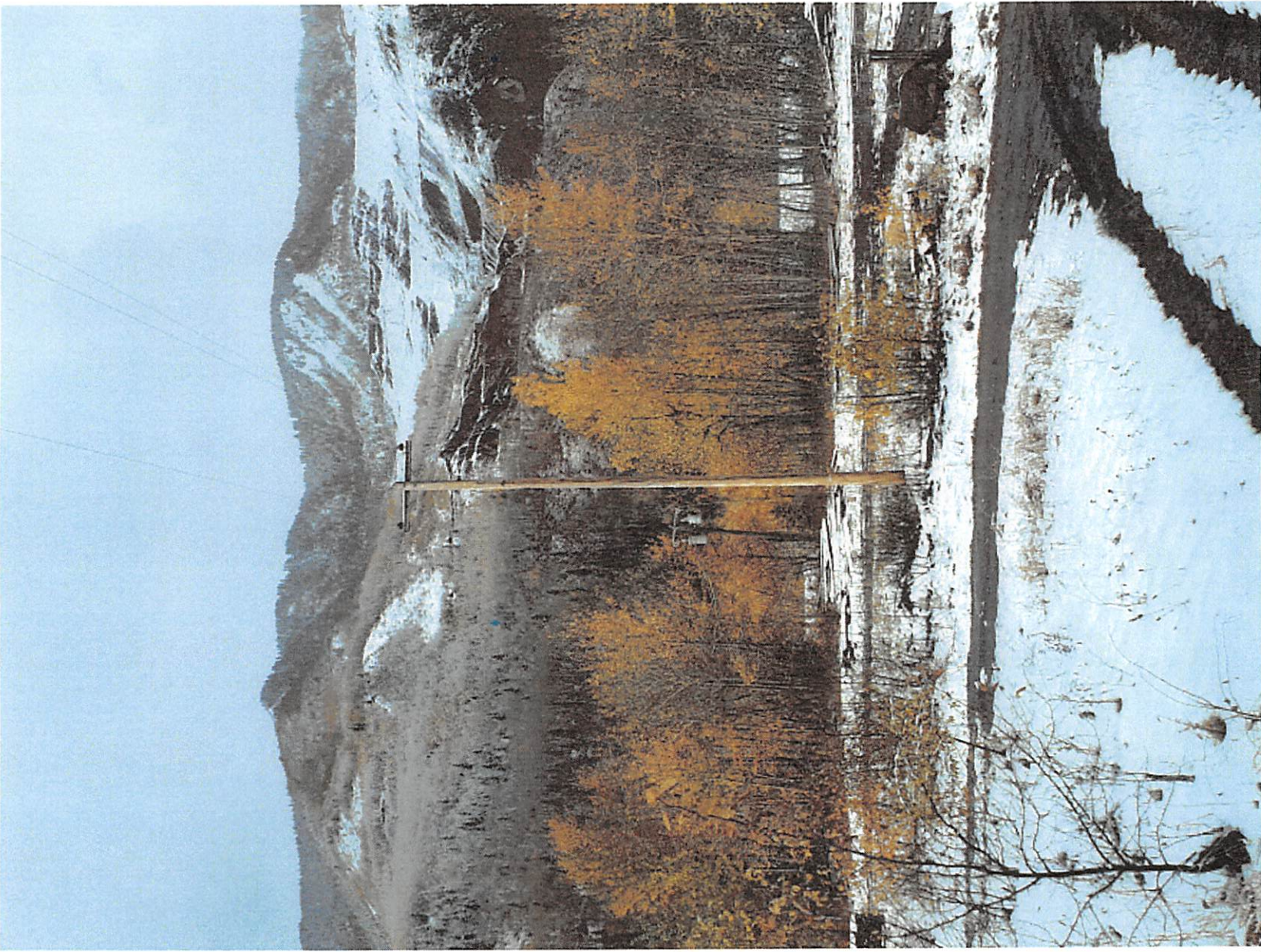
Photograph 4.a – power pole 585838 in the foreground and power pole 585839 with transformers in the background.
