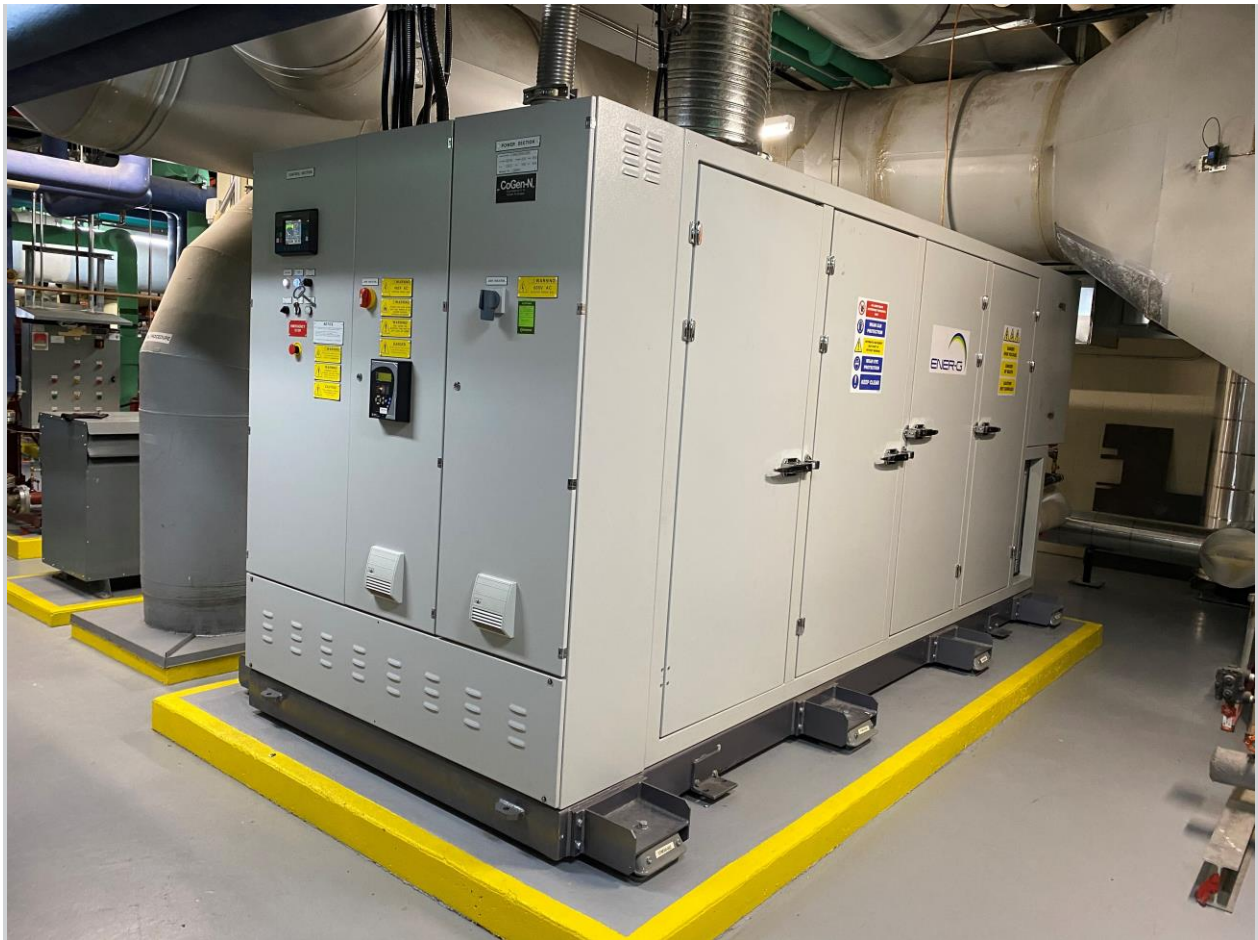
ATB Place's Co-Gen in North Tower 2
