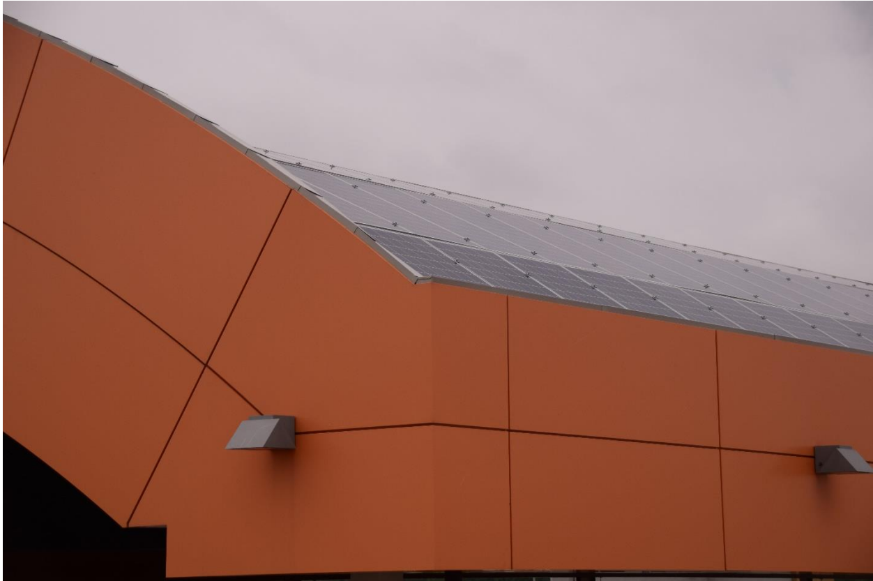
Figure 5: Solar panels installed on the roof of Sorensen Station in downtown Red Deer. Solar panels help reduce emissions from energy generation in the Red Deer Air Quality Management Area.
