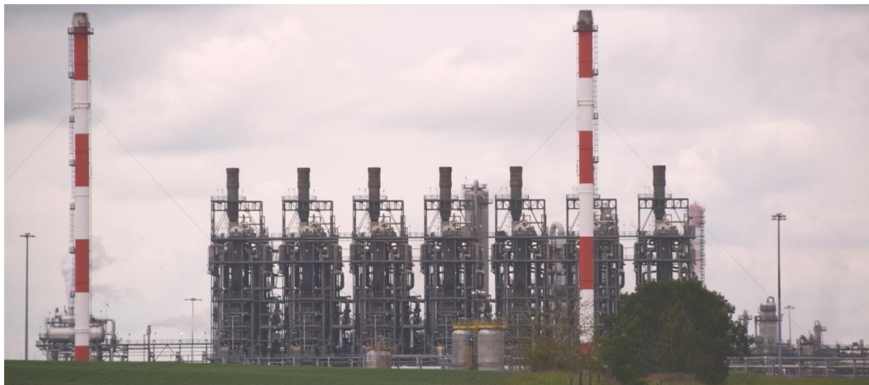
Figure 6: Ethylene cracking furnaces and flare stacks at NOVA Chemicals Corporation's Joffre Facility. NOVA Chemicals Corporation are refurbishing some ethylene cracking furnaces to reduce NO x emissions.
