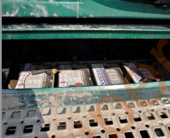
Battery and Battery Cable
