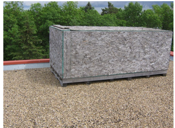
Negative pressure unit.
