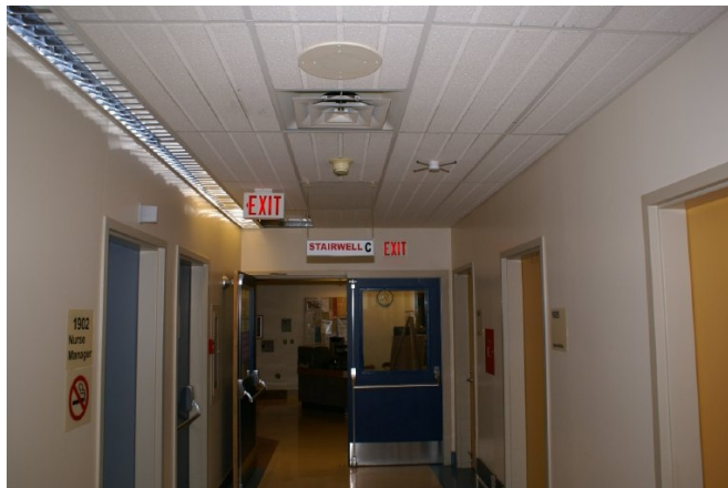
Typical exit signs in corridor
