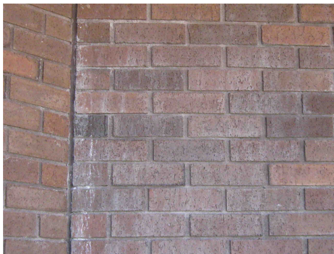
Cracked control joints at brick wall.
