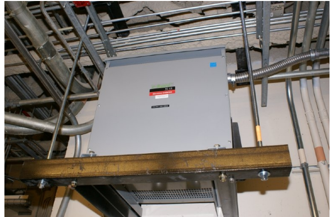
75KVA transformer ET2
