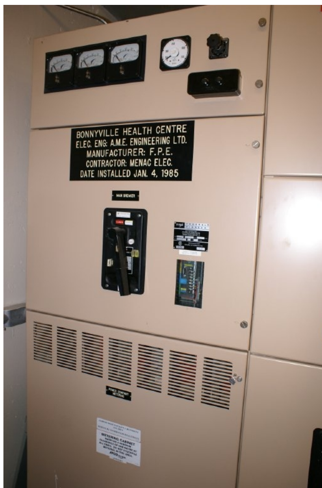
Main distribution switchgear
