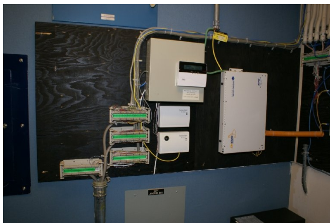
The main intrusion detection control panel
