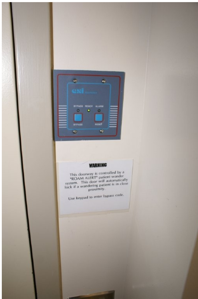
Patient wandering system control adjacent door to corridor.
