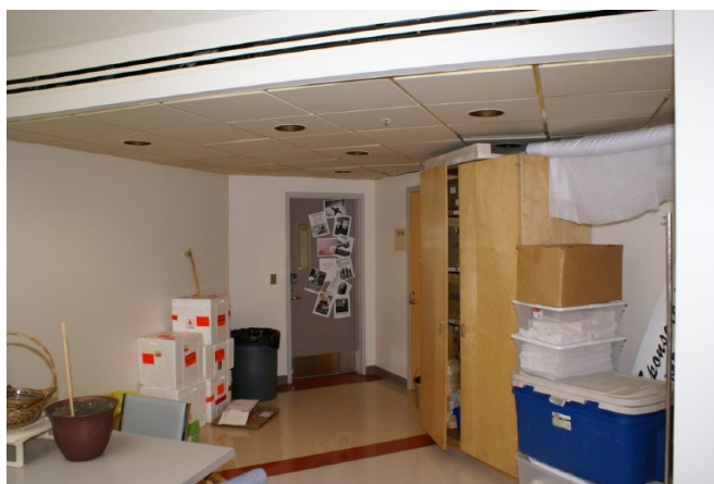
Incandescent downlighting in the 1998 reno area.
