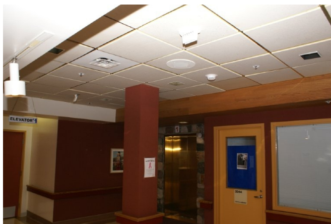
New fire alarm smoke detector in the elevator lobby.
