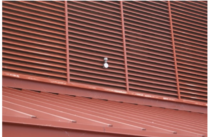
Exterior photocell on mechanical penthouse wall.
