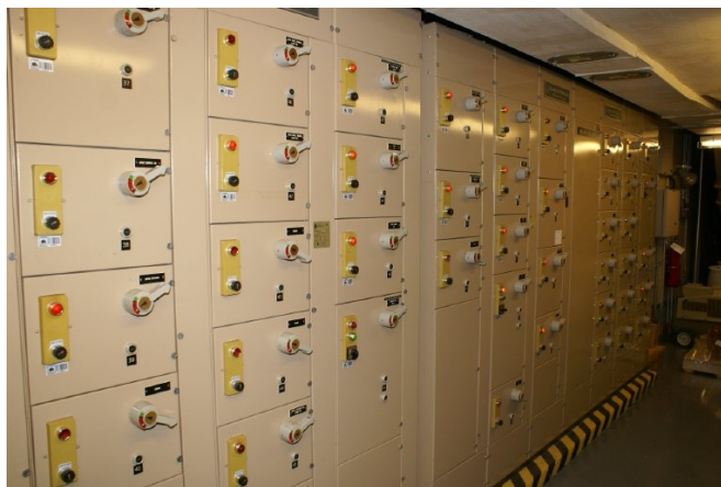
MCC #2 and MCC #E2
