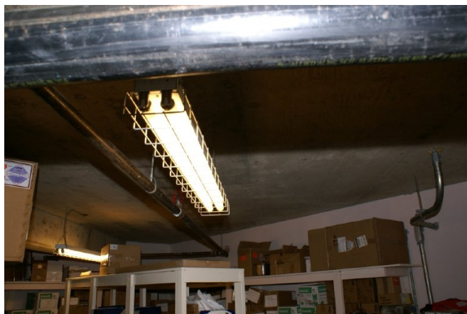
Typical fluorescent strip lights in the Lab basement
