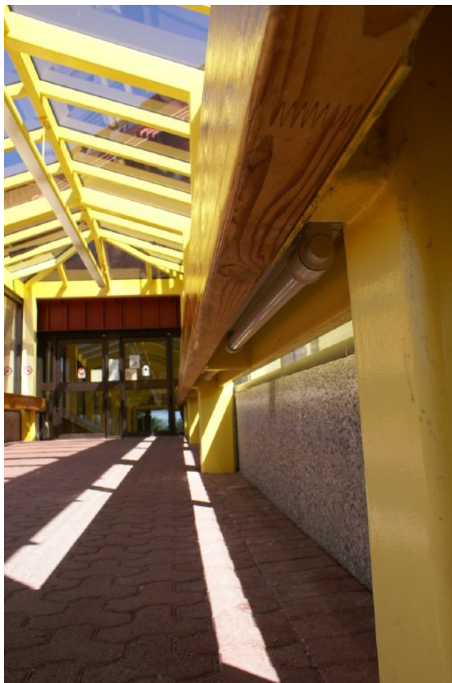
Exterior fluorescent fixtures mounted under handrails
