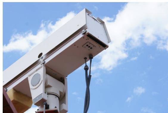
Damaged conduits feeding security camera.
