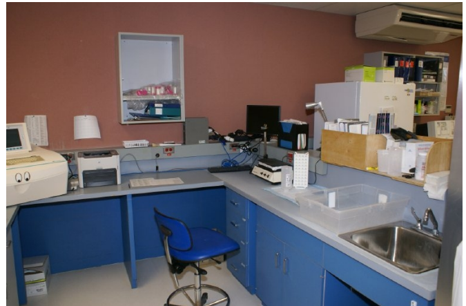
Dual channel raceway installed above counters.
