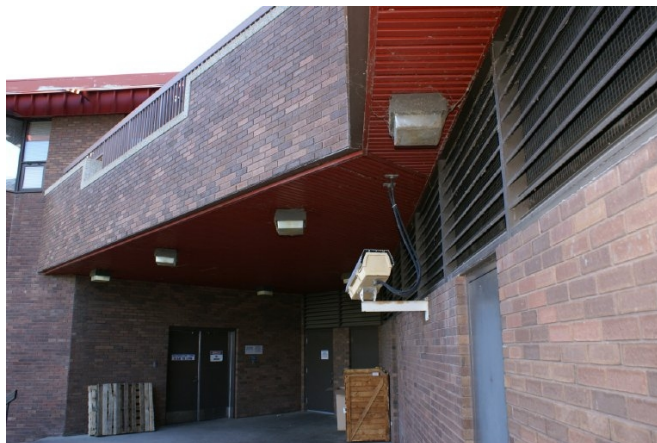
H.P.S. Canopy fixtures located at the loading dock
