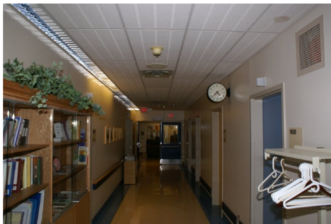
Typical fluorescent valance lighting in corridors
