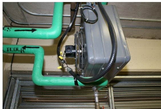
Improper wiring of unit heater in the generator room.
