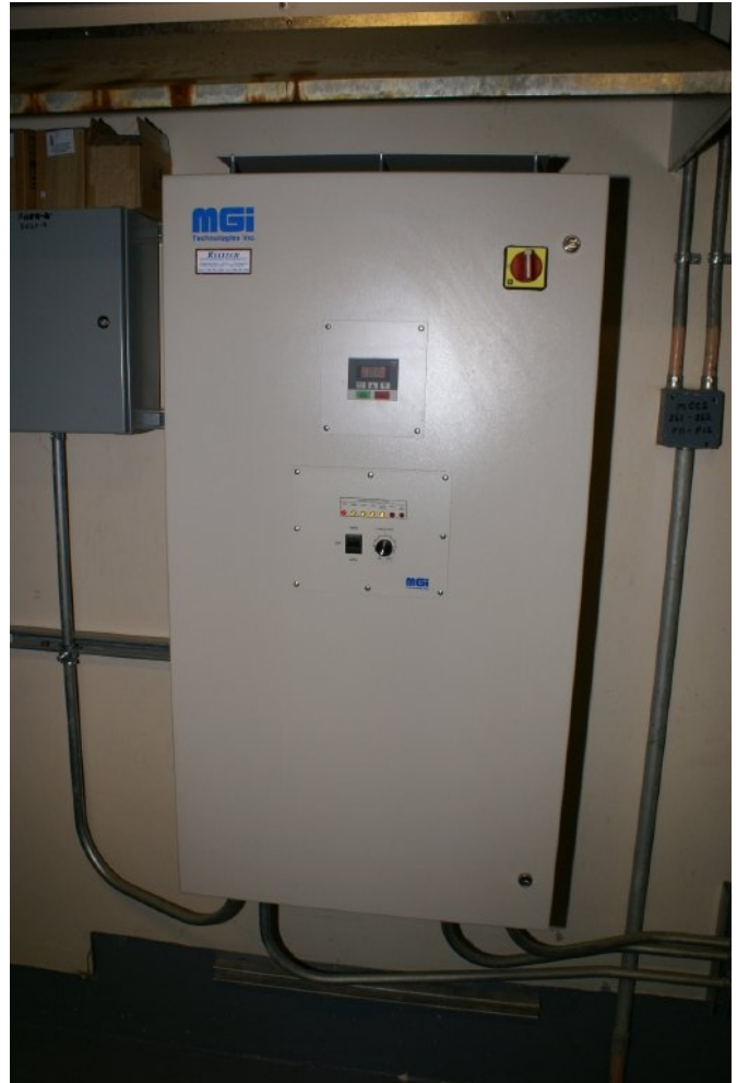
MGI Technologies VFD panel
