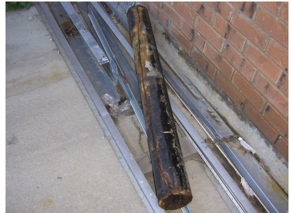
Cracked Sewer Pipe.
