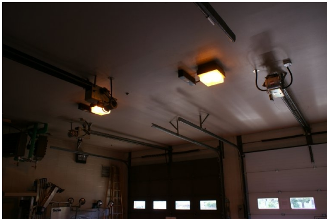
HID fixtures in the ambulance garage
