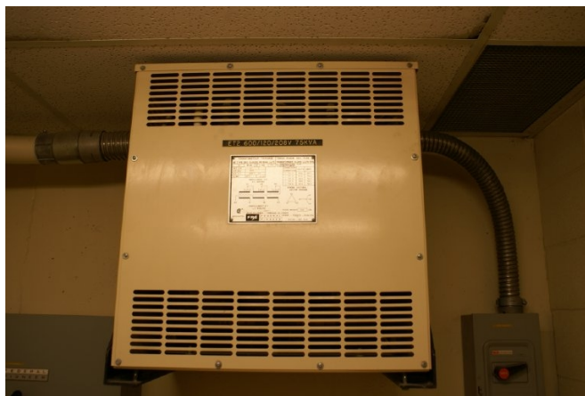
Typical federal pioneer transformer
