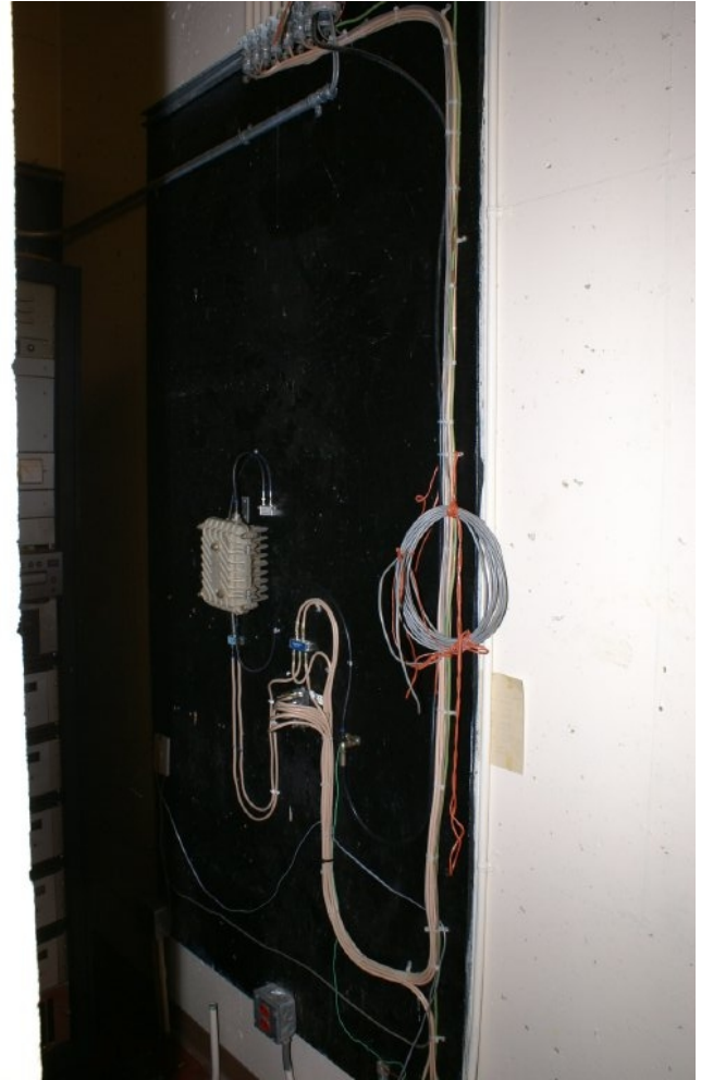
The main CATV demarcation
