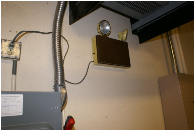
Emergi-Lite battery pack located in the main electrical room.
