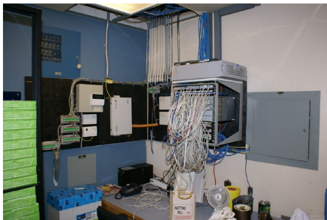
Data rack/patch panel located behind the main desk.
