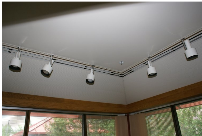
Typical incandescent track lighting
