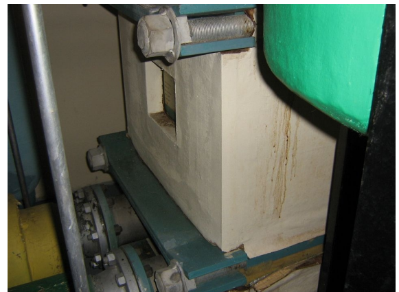
Domestic hot water heat exchanger.
