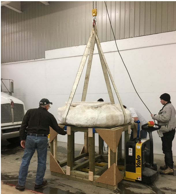
Figure 18. Positioning jacketed feature on temporary custom-built stand to facilitate construction of permanent legged base.
