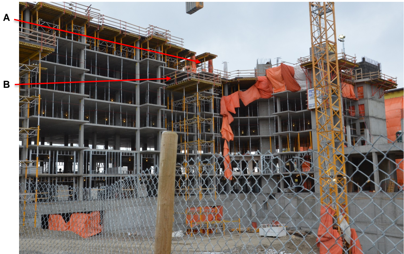
Figure 1. The south side of the building where the incident occurred.
