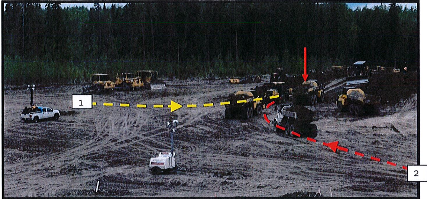
Photograph 3 – Shows an overview of the incident site. The arrow shows the approximate location of the incident.
