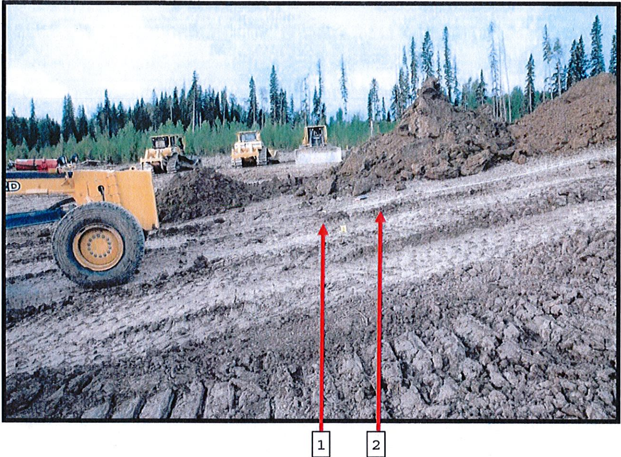
Photograph 6 – Shows a side view of the incident site.
