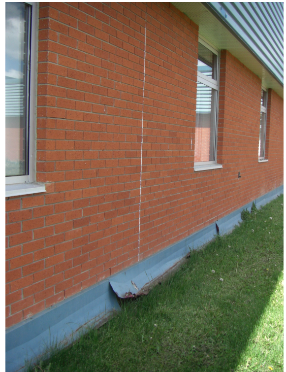
(1989) Original Building - has damaged prefinished metal skirting along foundation walls.
