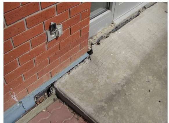
(Exit near Long Term Care - Exit at Vestibule 83) - has open gap of concrete slab along foundation wall.
