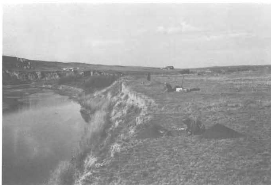
Figure 12: Looking west at excavation of Units 2, 3 and 4, Dg0v-94, above cutbank on north side of Milk River.
