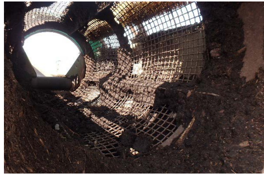
Photo 3.38. Clogging of trommel screen Source: CH2M
