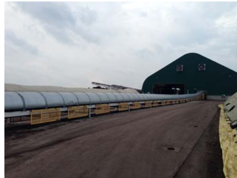
Photo 3.39. Using horizontal conveyors to move material over longer distances can reduce operating costs compared to using front-end loaders
