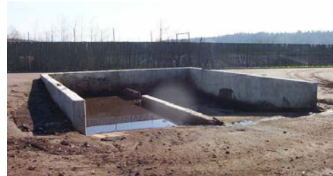
Photo 4.38. Basins and intercepts can be used to keep sediments out of retention ponds
