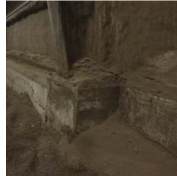
Photo 4.25. Dust that accumulates in buildings can be a fire hazard
