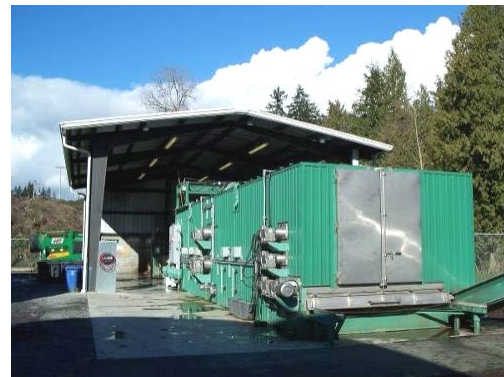
Photo 3.22. Agitated container system composting system
