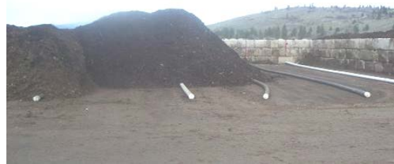
Photo 3.10. Typical ASP system with aboveground piping
