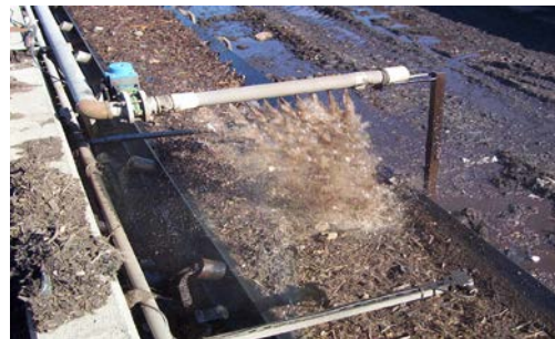
Photo 4.15. Spray bar installed on a horizontal conveyor
