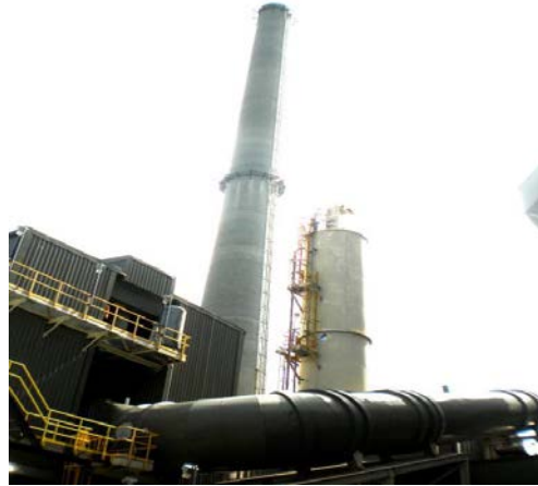
Photo 1.13. Waste-to-Energy facility Source: JLT Technical Services
