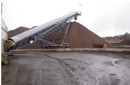
Photo 3.40. Radial stacking conveyor used to make a large linear stockpile
