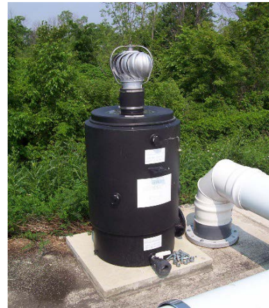
Photo 4.32. Carbon adsorption systems can be used to treat odours on sumps and tanks
