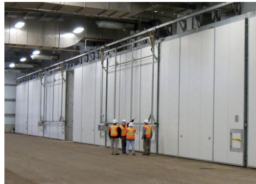
Photo 3.24. Doors on tunnel composting system
