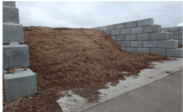
Photo 4.13. Material at the bottom edges of an ASP pile is not likely to reach the temperatures needed for pathogen reduction. Turning the ASP “inside-out” at least once during active composting helps prevent pathogen regrowth
