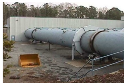
Photo 3.26. Large-scale drum composting system
