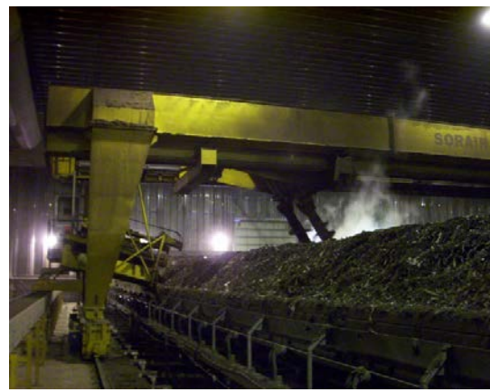
Photo 3.20. Bridge crane and suspended auger turning mechanism in Edmonton, AB viewed from discharge side of bay
