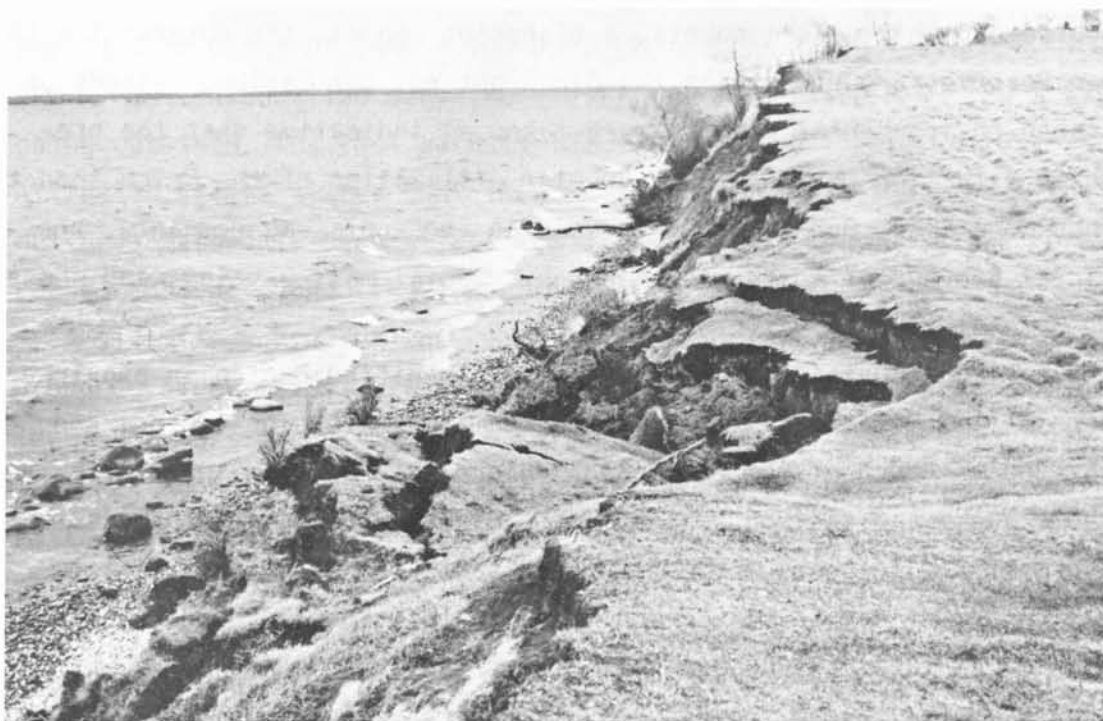
Figure 27: Typical erosional feature (Maccagno's Point). North side shooting east.
