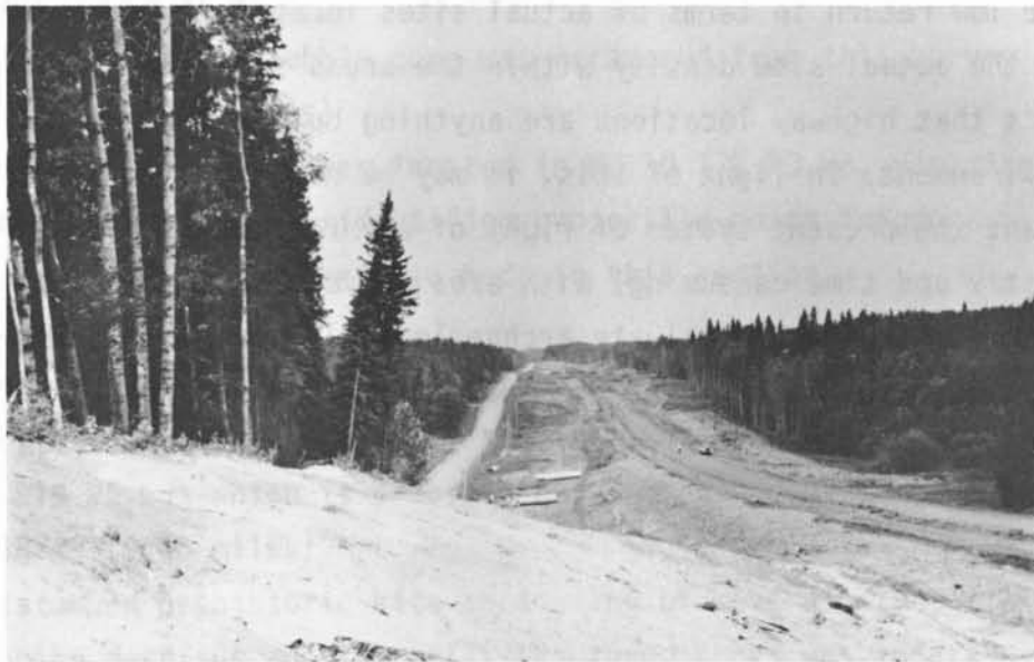
Figure 9: A general view north along Project 2:44 right of way across Lawrence Lake basin.
