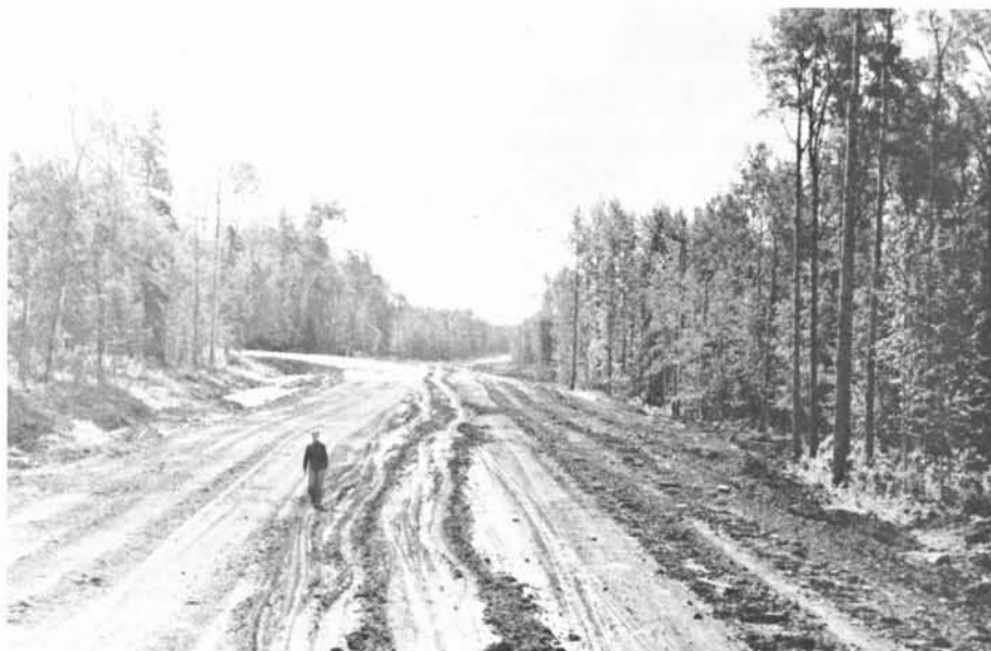
Figure 10: A general view south of Project 967:02 right of way clearing near Marten Tower Road.
