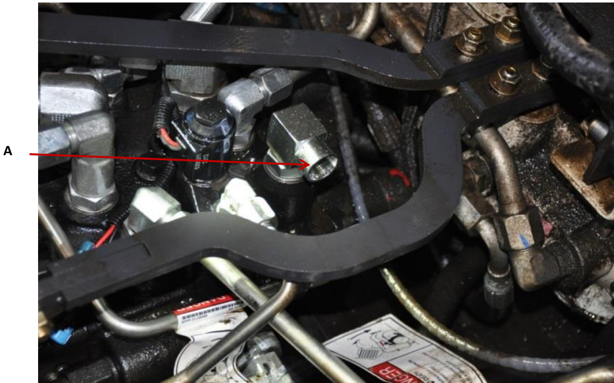
Figure 6. The mechanic had removed the suspected leaking lift circuit line off the control valve. A: The control valve fitting.
