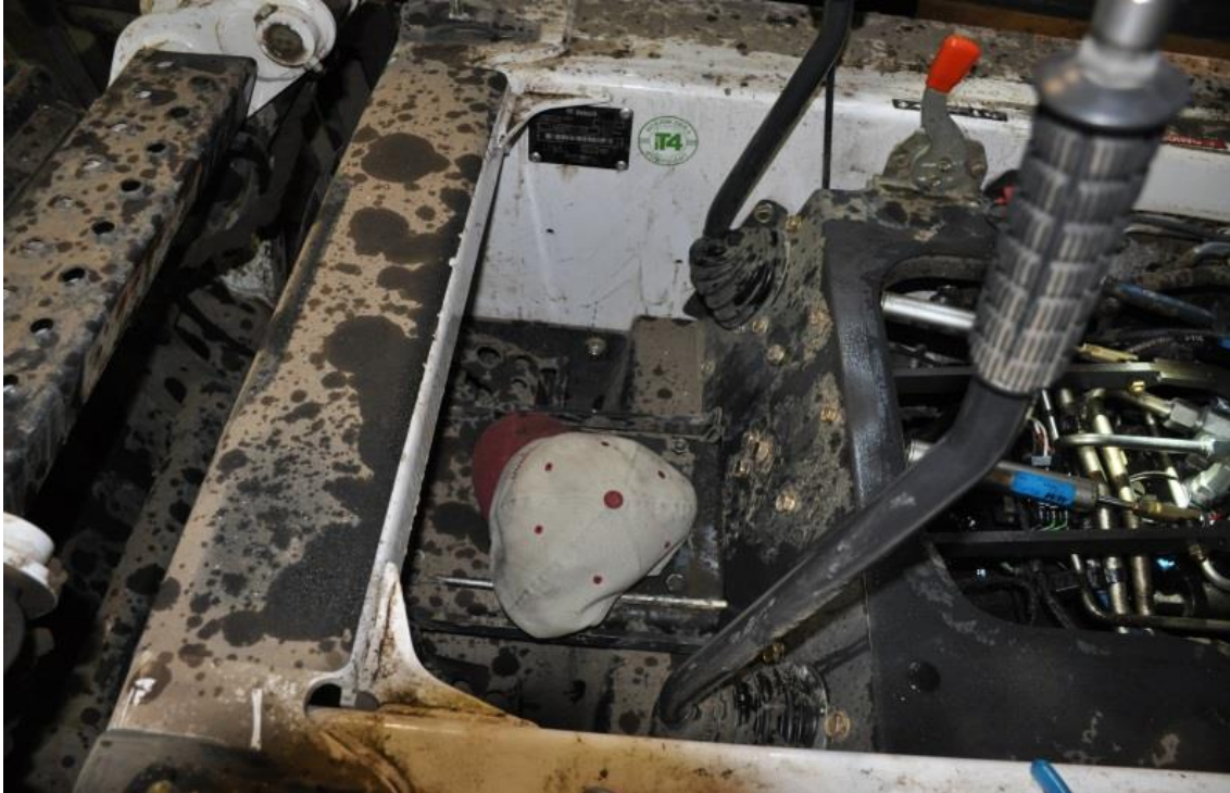
Figure 7. The sprayed hydraulic oil inside the motor compartment from the loosened hose.
